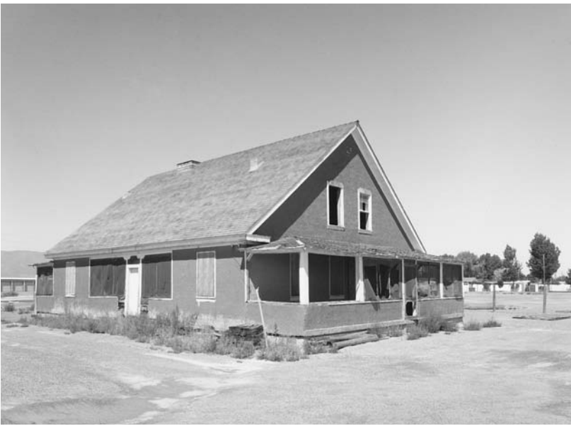
The Marvel Ranch cookhouse, built in 1920, is an excellent expression of the type of architecture that once dominated the rural parts of the state.
