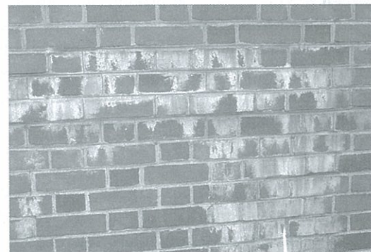
Figure 39. Typical white efflorescent salts on brick masonry.
