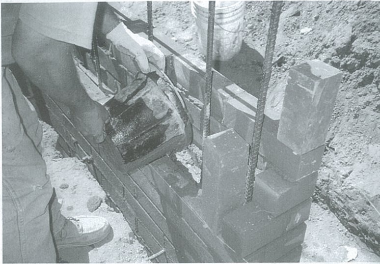
Figure 20. Pouring grout. Note ideal squeeze-out of mortar in back wall. See pages 42-50 construction procedure.
