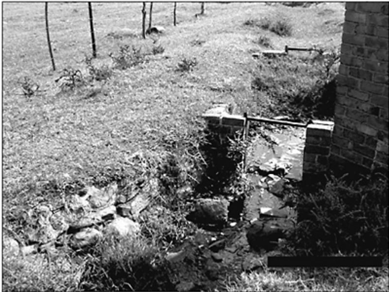
Figure 8.4. Distribution chamber and open ditch at Crowborough farm.
