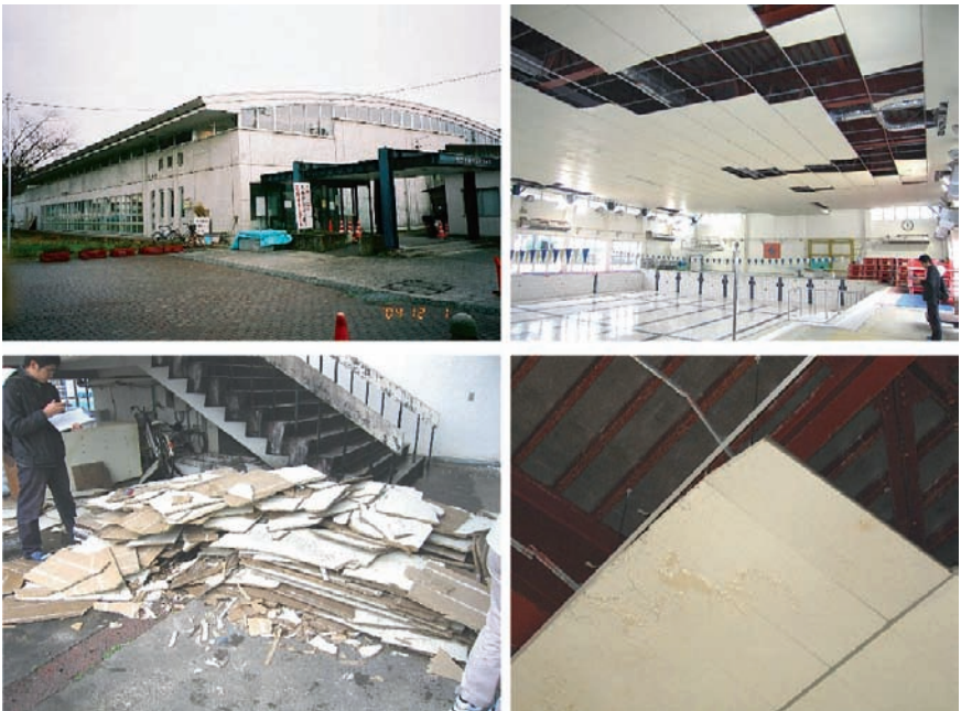
Fig. 9-30. Damage to ceiling systems in a swimming pool
