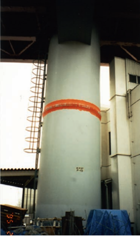
Fig. 8-9. Buckling of steel pier of circular hollow section
