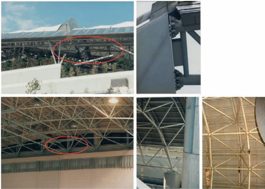
Fig. 9-12. Failed members of space frames
