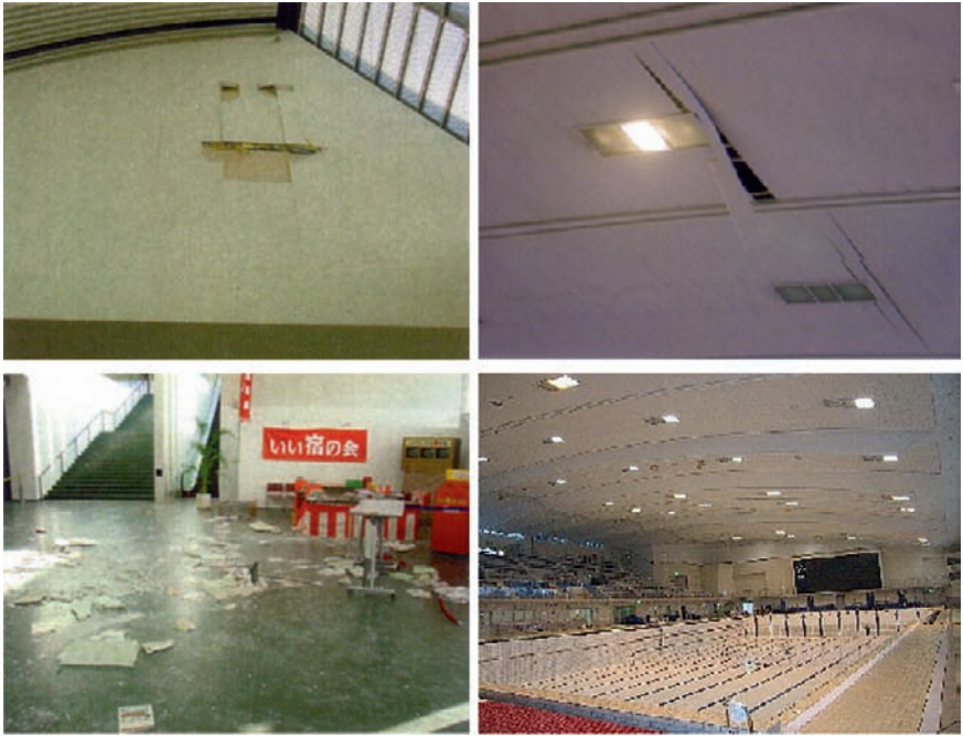
Fig. 9-31. Damage to nonstructural components during Fukuoka earthquake
