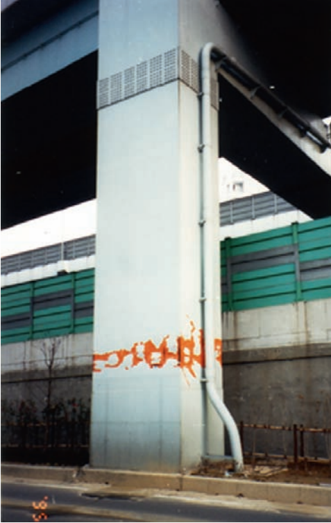
Fig. 8-8. Buckling of steel pier of rectangular hollow section
