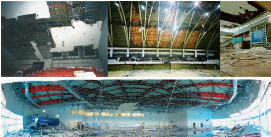
Fig. 9-24. Examples of damage to suspended ceilings
