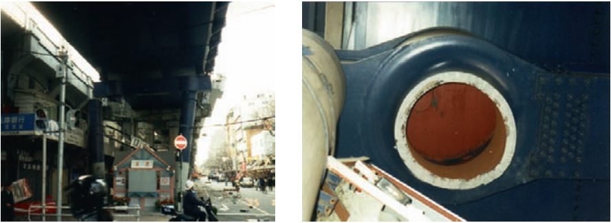
Fig. 8-11. Buckling of steel pier of centrifugally cast steel pipe
