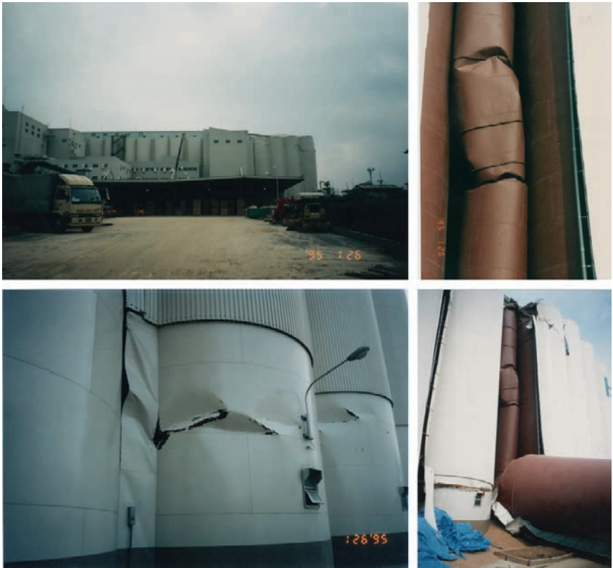
Fig. 9-9. Silos damaged by Kobe earthquake
