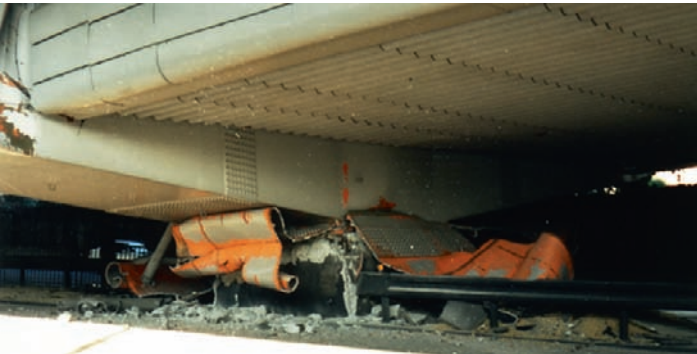
Fig. 8-10. Collapse of steel pier of rectangular hollow section
