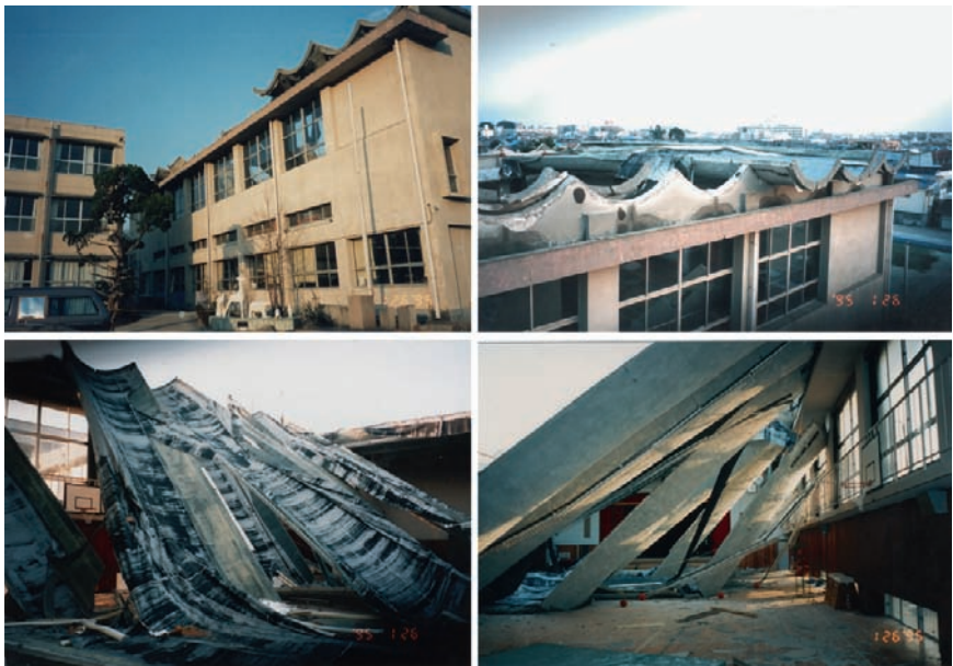
Fig. 9-16. View of the school gymnasium with a precast beam roof after the earthquake
