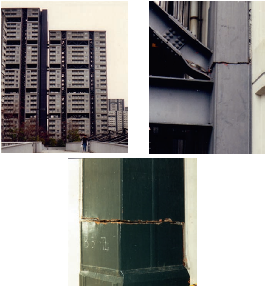
Fig. 8-6. Brittle fracture of columns in a mega-structure
