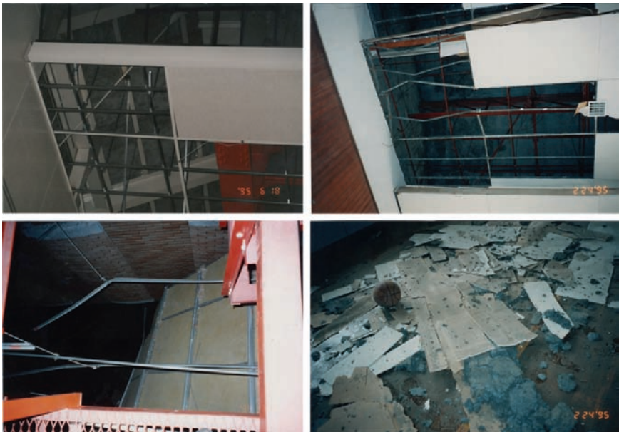
Fig. 9-20. Damage to suspended ceilings
