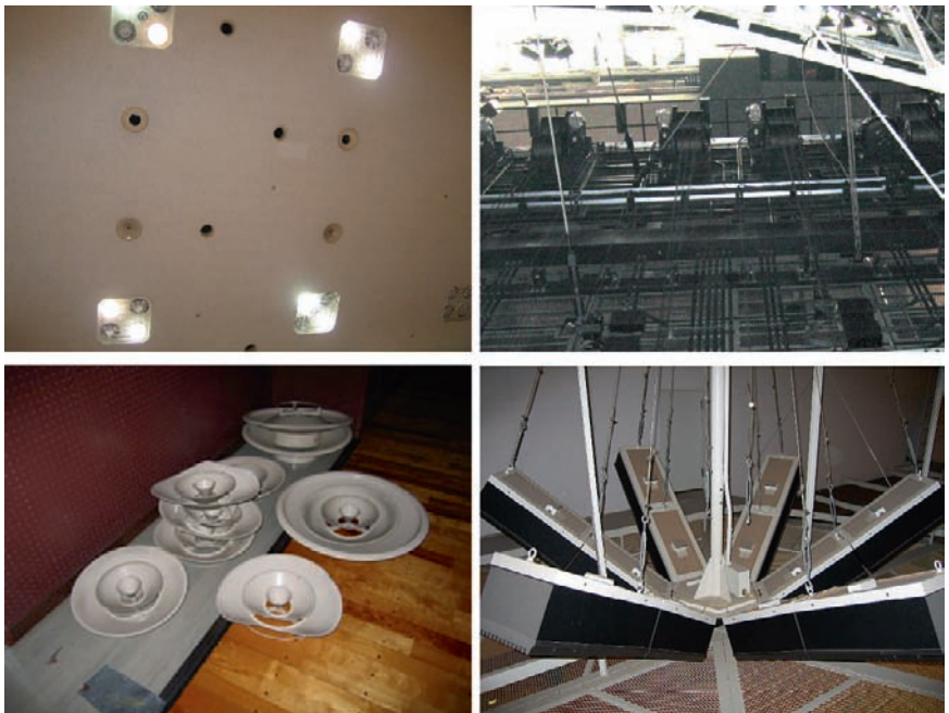
Fig. 9-32. Damage to facilities settled in the heights during Fukuoka earthquake
