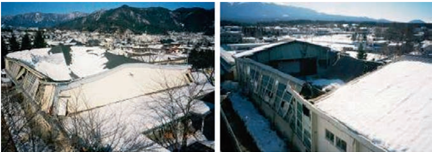
Fig. 9-2. Wide-roof gymnasiums collapsed under heavy snow
