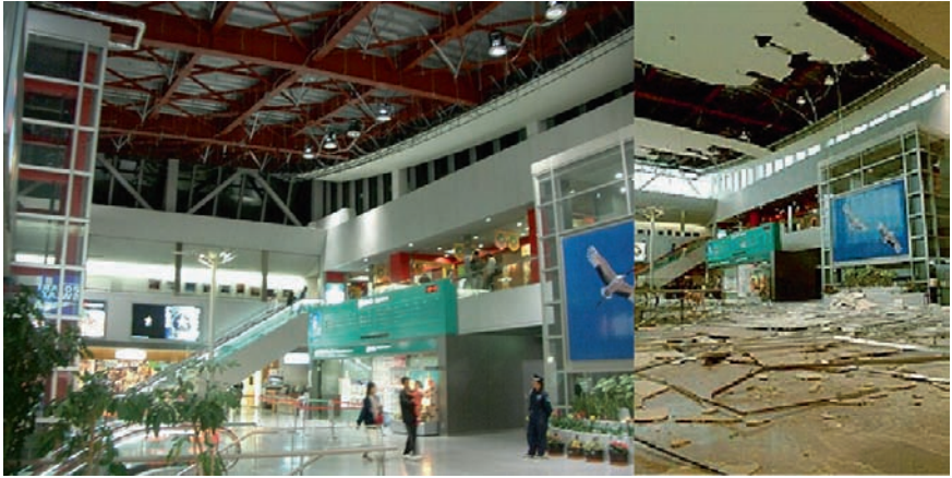
Fig. 9-26. Damage to the ceiling in Kushiro airport terminal
