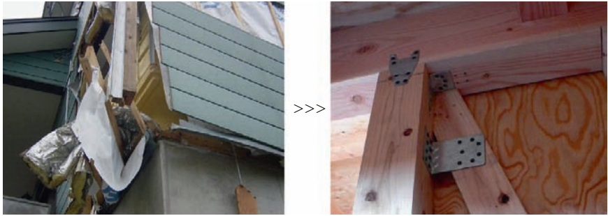
Fig. 10-8. Insufficient joint around the bearing wall
