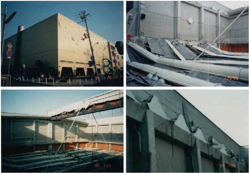
Fig. 9-18. View of the public gymnasium with a precast beam roof after the earthquake
