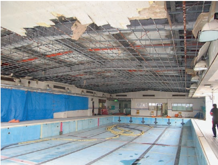
Fig. 9-36. Sudden collapse of ceilings with no earthquake in a swimming pool in Saitama
