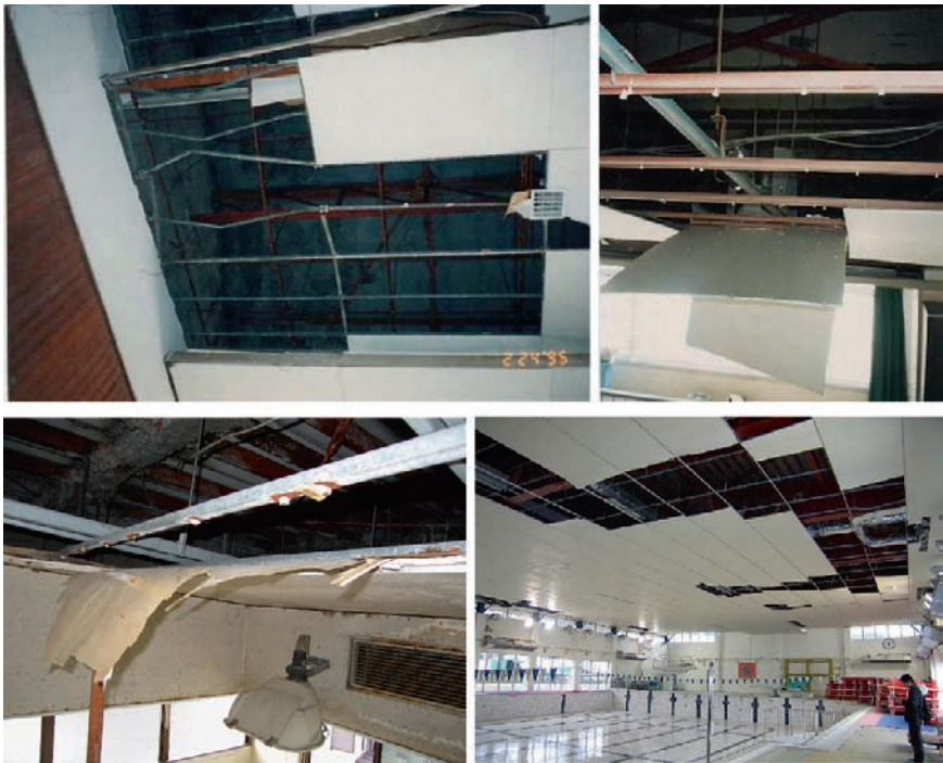
Fig. 9-35. Various types of failure of ceiling systems
