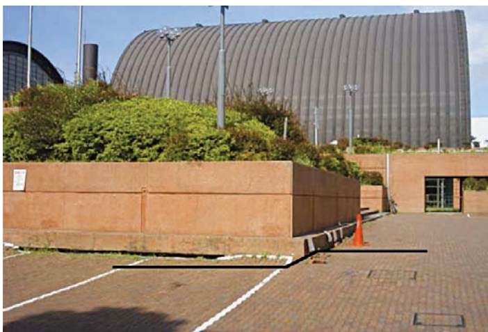
Fig. 14-8. Damage in building due to subsidence of landfill
