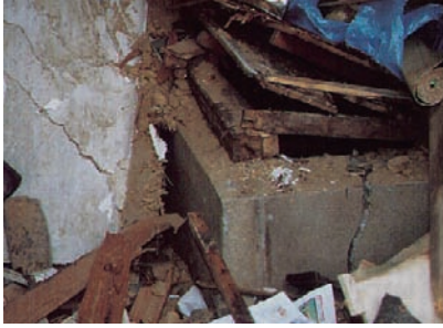
Bending Failure of not Reinforced Concrete Foundation
