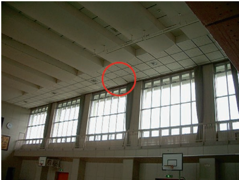
Fig. 9-25. Miyagi-ken earthquake (Courtesy of Dr. Y. Sakai)
