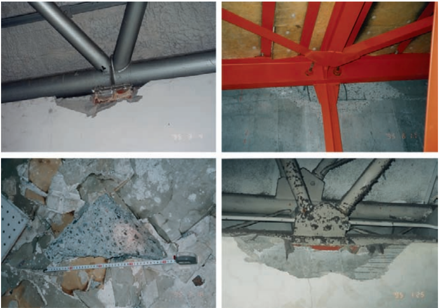
Fig. 9-11. Failure at bearings of supporting structure for roof frames
