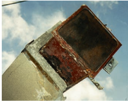
Fig. 8-4. Overturn of a four-storey steel office building
