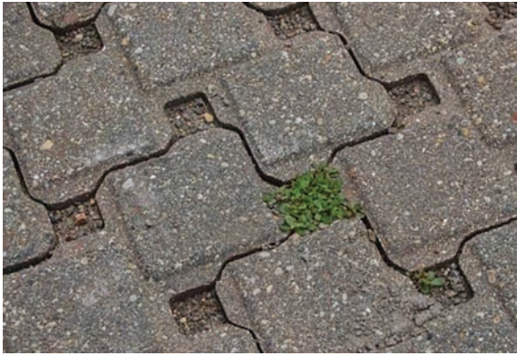
Figure 8-12 Before vacuum cleaning of a PICP parking lot surface that was not cleaned for seven years Source: ICPI
