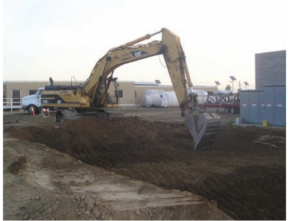
Figure 2-15 Excavator operating from outside the excavation to prevent compaction of subgrade, Modesto, CA
