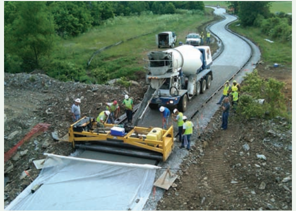
Figure 3-20 Finishing performed with a power-roller screed, Legacy Recreational Trail, Lexington, KY Source: Concrete Promotional Group, Inc.
