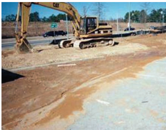
Figure 3-23 Erosion and sediment control failure, GA
