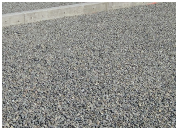
Figure 7-3 Aggregate base/subbase for this porous asphalt pavement is clean and free of fines, Waste Management Woodinville, Woodinville, WA
