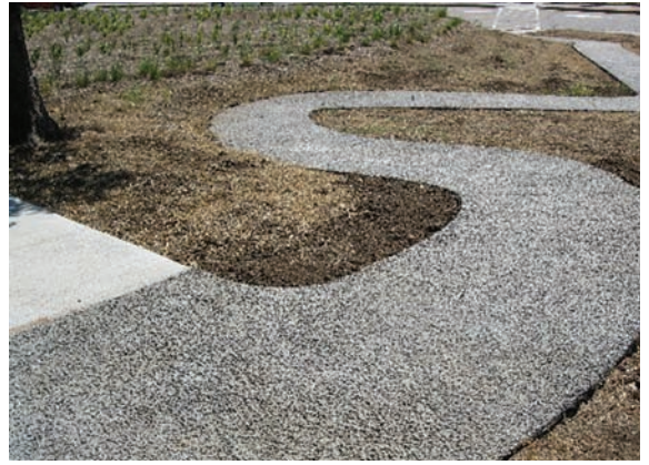
Figure 3-5 Pervious concrete sidewalk at the Johnson County Community College, Overland Park, KS Source: Concrete Promotional Group, Inc.
