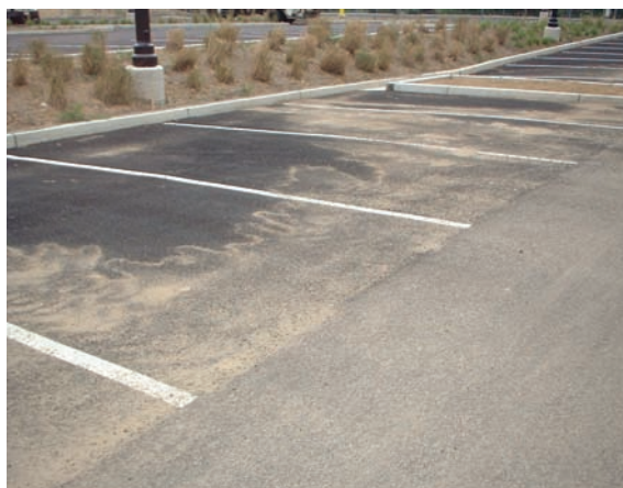
Figure 8-1 Porous asphalt pavement clogged by runoff sediments from an unstabilized adjacent area, Philadelphia, PA
