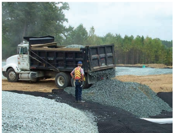
Figure 2-19 Aggregate placed in the bed from the edge to prevent compaction, Chapel Hill, NC
