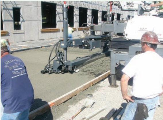
Figure 3-21 Industrial loading dock. Finishing performed with a pervious concrete laser screed, Lacey, WA Source: Puget Sound Concrete Specification Council
