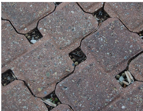
Figure 8-4 Organic material deposition in PICP openings from nearby trees Source: NCSU
