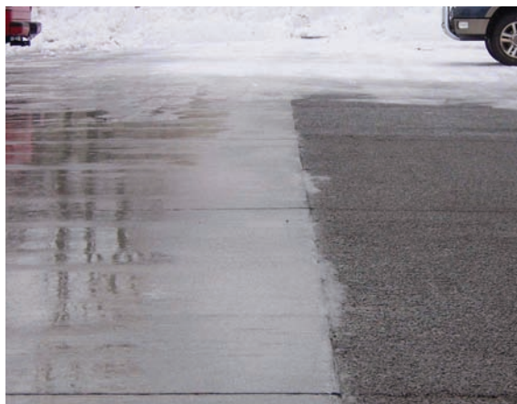
Figure 3-14 Standard concrete adjacent to pervious concrete in cold climate, Iowa State University, Ames, IA Source: John Kevern
