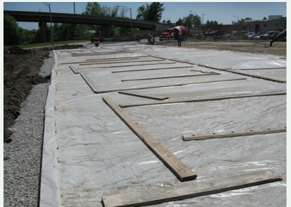
Figure 3-22 Plastic sheeting secured on the pervious concrete, Overland Park, KS Source: Concrete Promotional Group, Inc.
