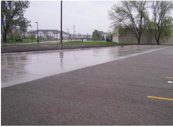
Figure 3-4 Pervious concrete adjacent to traditional concrete during a rainfall, Ames, IA Source: John Kevern
