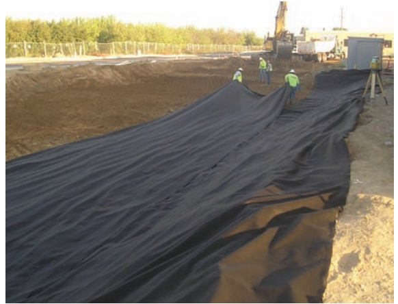
Figure 2-17 Geotextile being placed by hand to avoid compaction of subgrade, Modesto, CA
