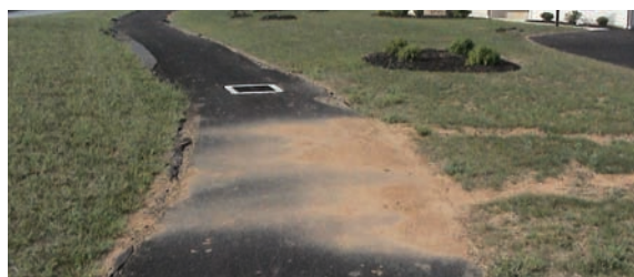
Figure 2-22 Sediment-laden stormwater runoff clogs the porous asphalt, Campbelltown, PA Source: CH2M HILL
