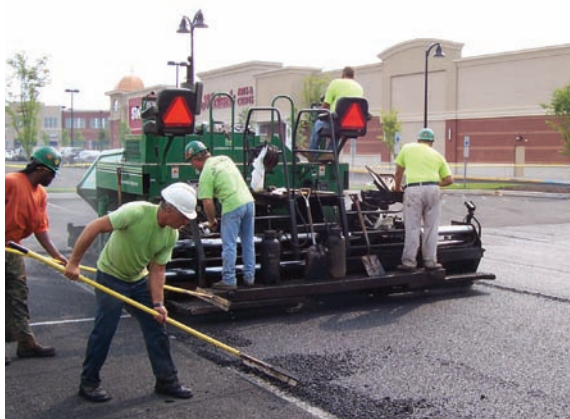
Figure 2-20 Installation of porous asphalt over the aggregate base layer with a tracked paver, Warrington, PA Source: CH2M HILL
