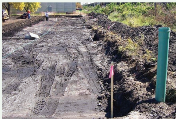
Figure 3-15 Excavation of base for aggregate storage layer prior to scarification and placement of geotextile fabric, Ames, IA
