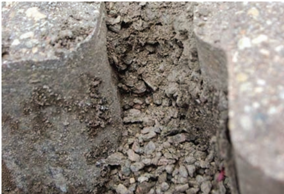
Figure 8-14 PICP opening showing trapped sediment at the top with aggregate under it Source: NCSU
