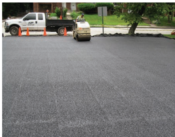
Figure 2-21 A small roller smooths seams of porous asphalt surface course, Yeadon, PA Source: CH2M HILL
