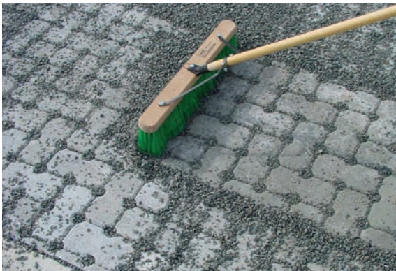
Figure 8-16 Replacement is simple and done with a broom or with mechanical sweepers for larger areas. Source: NCSU
