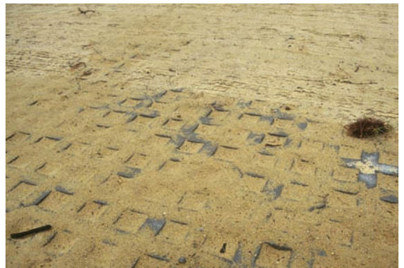
Figure 8-17 Hollowed out concrete grid pavement voids penetrated by mechanical sweeper bristles, leaving loose sand from large voids on pavement surface to be swept back into voids. Source: NCSU
