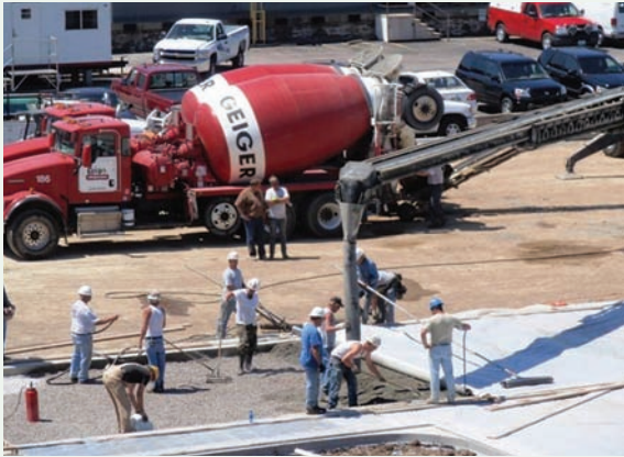
Figure 3-19 Concrete deposited as close as possible to the final location. Finishing performed with a hydraulic roller screed, Overland Park, KS Source: Concrete Promotional Group, Inc.
