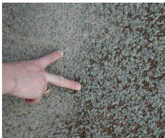
Figure 8-6 Visual inspection of a pervious concrete lot shows sediment and leaf debris accumulation
