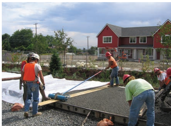
Figure 7-5 Installation of this pervious concrete roadway takes careful planning, High Point Redevelopment Phase 1, Seattle, WA
