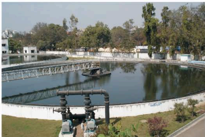
Primary Sedimentation Tank
