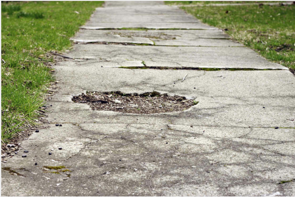
Sidewalks in disrepair.
