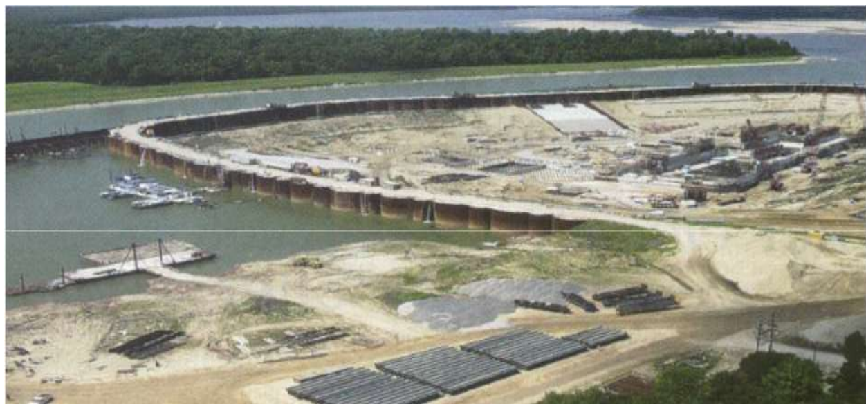
Figure 5.21 Sheet-piling used to divert a river while building a dam and locks on the White River in Arkansas
