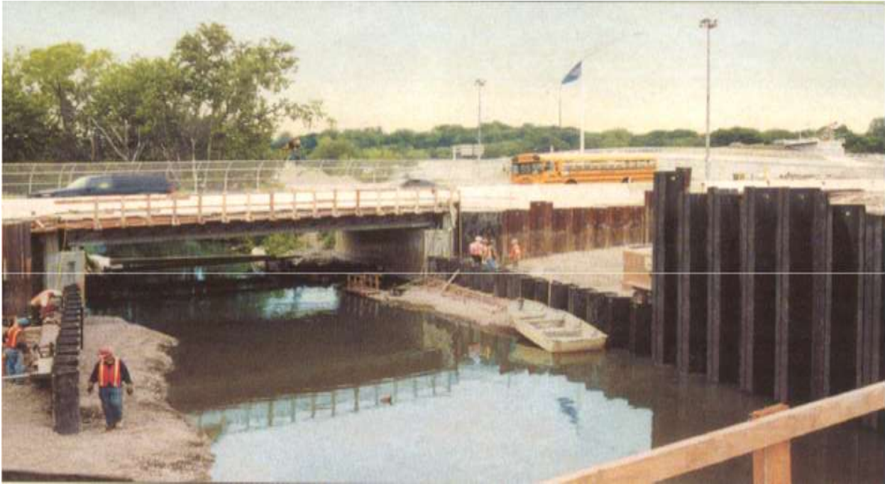
Figure 5.19 Sheet piling used to expand a bridge's width, while maintaining highway and river traffic
