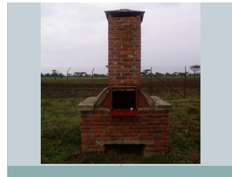
Low temperature incinerator
