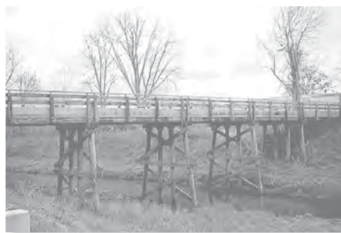
Influence lines for the continuous girder of this trestle were constructed in order to properly design the girder.
