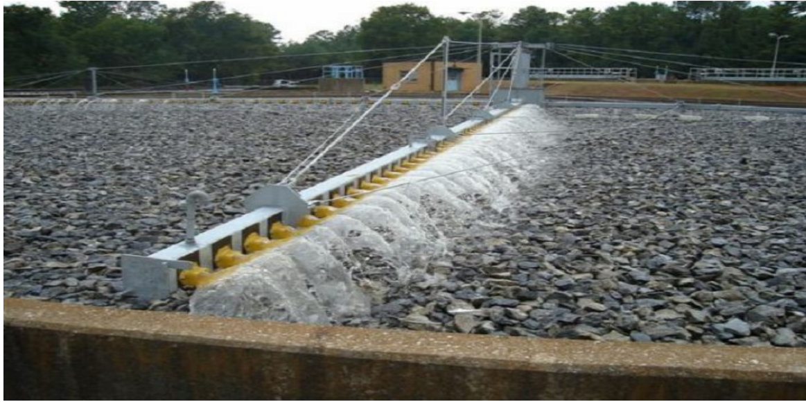
Figure: - Photographic view of rotary distributors
