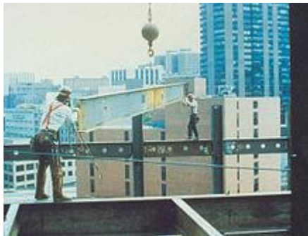
At-risk workers without appropriate safety equipment
