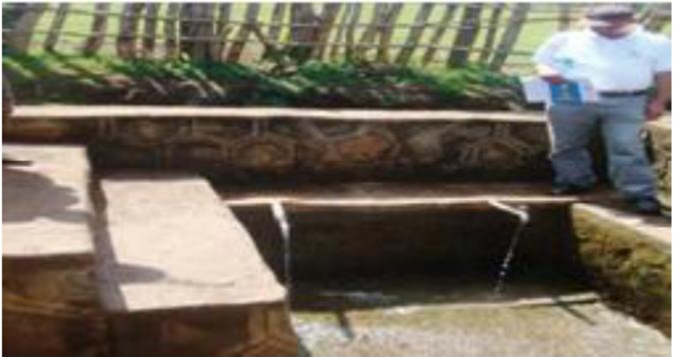
Figure 7.4: A protected spring. Note the concrete retention wall with two delivery pipes and the surrounding fence.
