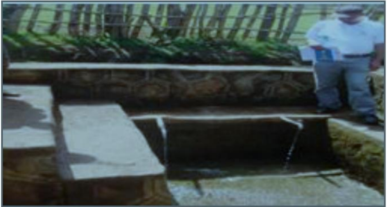
Figure 9.5:- A protected spring, Note the concrete retention wall with two delivery pipes and the surrounding fence.
