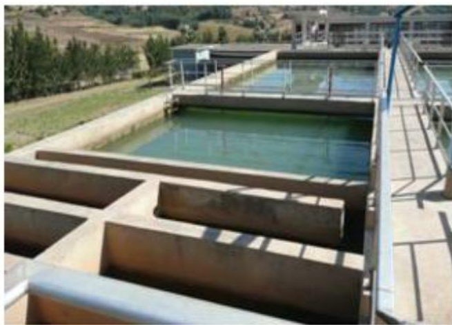
Figure 6.9: Sedimentation tank at a municipal water treatment works.
