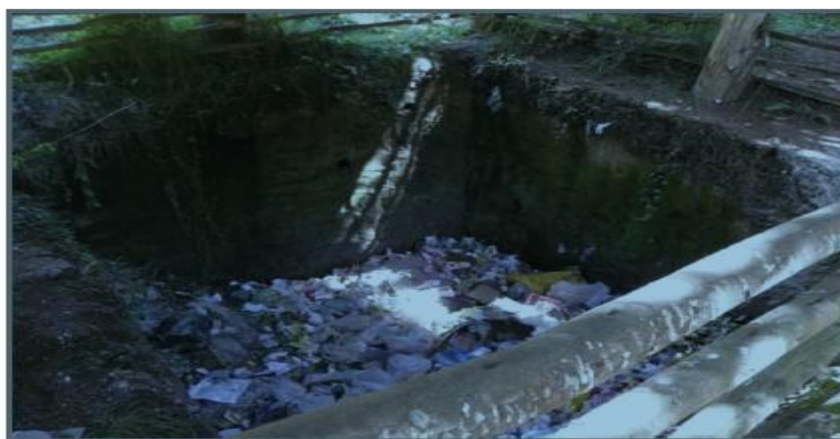
Figure 3.7:- Refuse pit with a fence to prevent people or animals from accidentally falling in.
