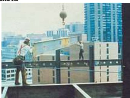
At-risk workers without appropriate safety equipment
