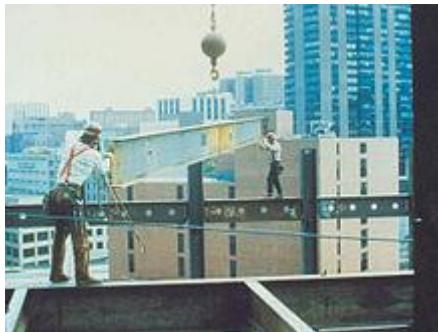
At-risk workers without appropriate safety equipment
