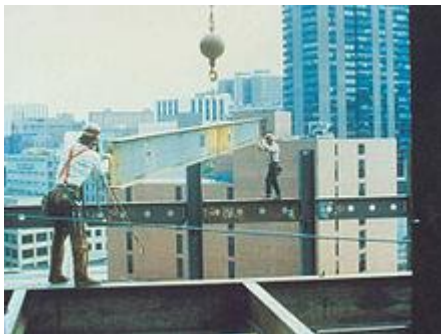
At-risk workers without appropriate safety equipment
