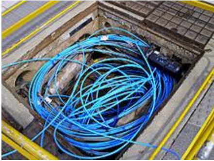
Fig.10 Single-mode optical fiber in an underground service pit
