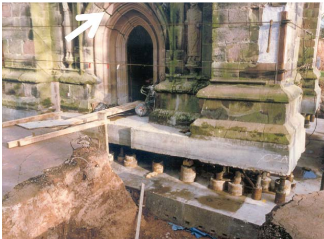
View of west side showing “fracture”
