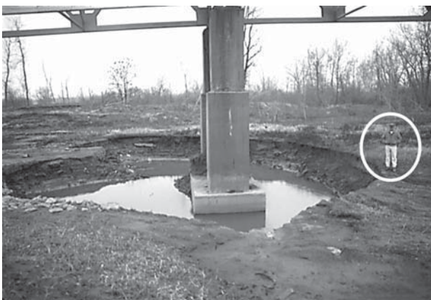
Figure 23.16 Scour hole around bridge pier.
