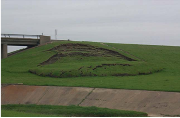
Figure 19.30 Shallow slide in a compacted embankment. (Courtesy of Professor Charles Aubeny, Texas A&M University.)
