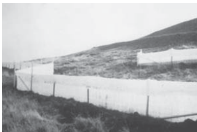
(a) Silt fences
