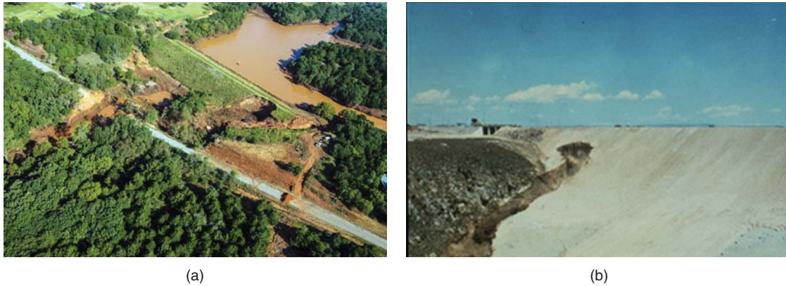
Figure 23.48 Internal erosion of an earth dam. (a) Blackman Creek Dam. (b) Teton Dam. (a: Photograph by Mark S. Harrison, Oklahoma Conservation Commission. Used by permission. b: Courtesy of Eunice Olson.)
