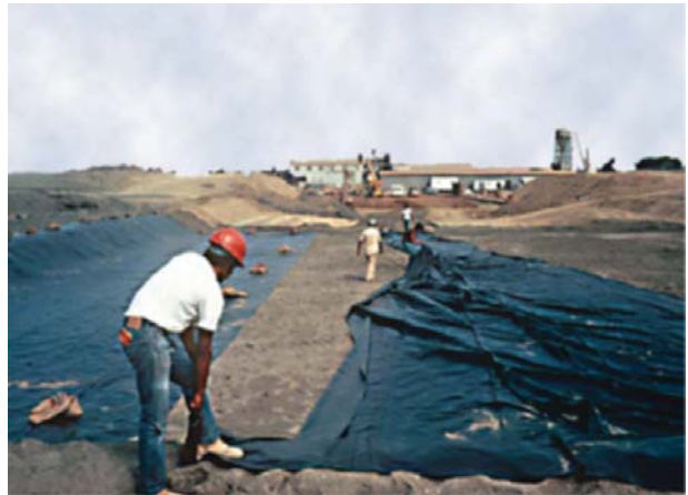
Figure 24.22 Installing a geomembrane in a bottom liner. (Courtesy of Layfield Environmental Systems, Layfield Group Limited, 11120 Silversmith Place, Richmond, British Columbia, Canada V7A 5E4.)
