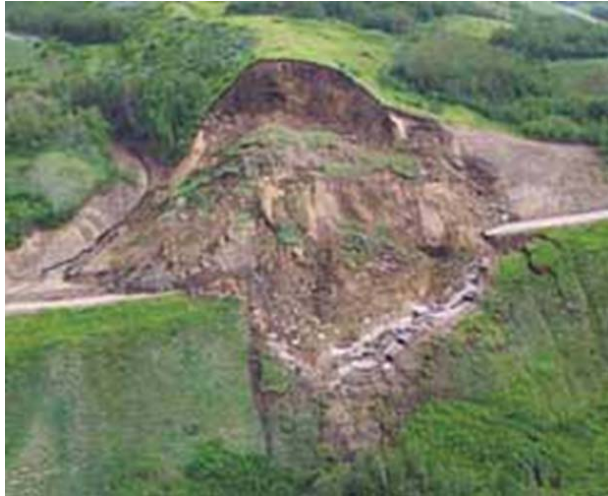
Figure 19.33 Three-dimensional slope failure. (Courtesy of Gordon W. Hunter, British Columbia Ministry of Transportation and Infrastructure.)
