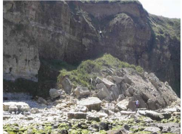
Figure 5.14 Massive collapse of rock cliff at Pointe du Hoc.
