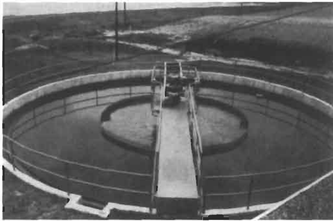
Figure 9-7. Circular settling tank.
