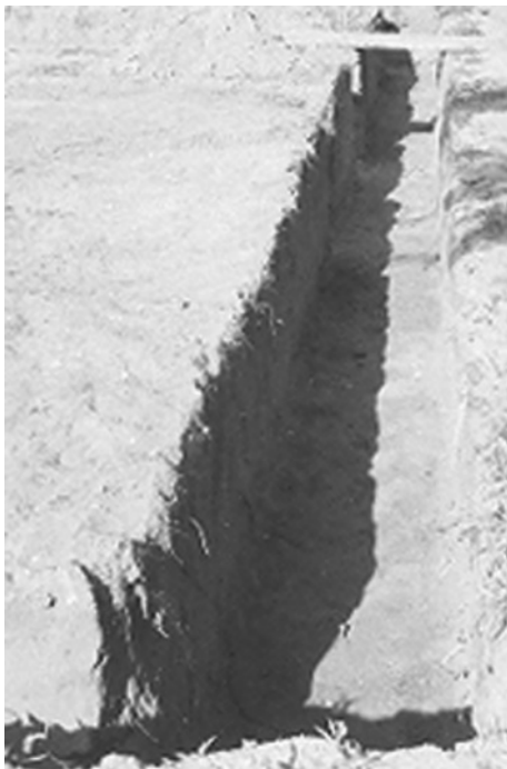
Figure 29.21 Excavation with sides of stable cemented sand (aeolian deposits) during the wet season in semi-arid conditions © A. Royal
