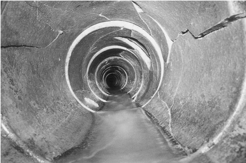
Fig. 17.2 CCTV image of a sewer in poor condition (courtesy of Telespec Ltd, Guildford)
