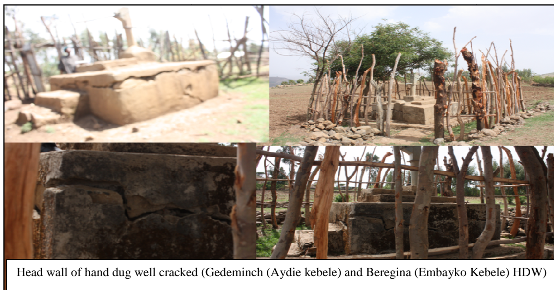
Figure 10: Cracked hand dug wells
