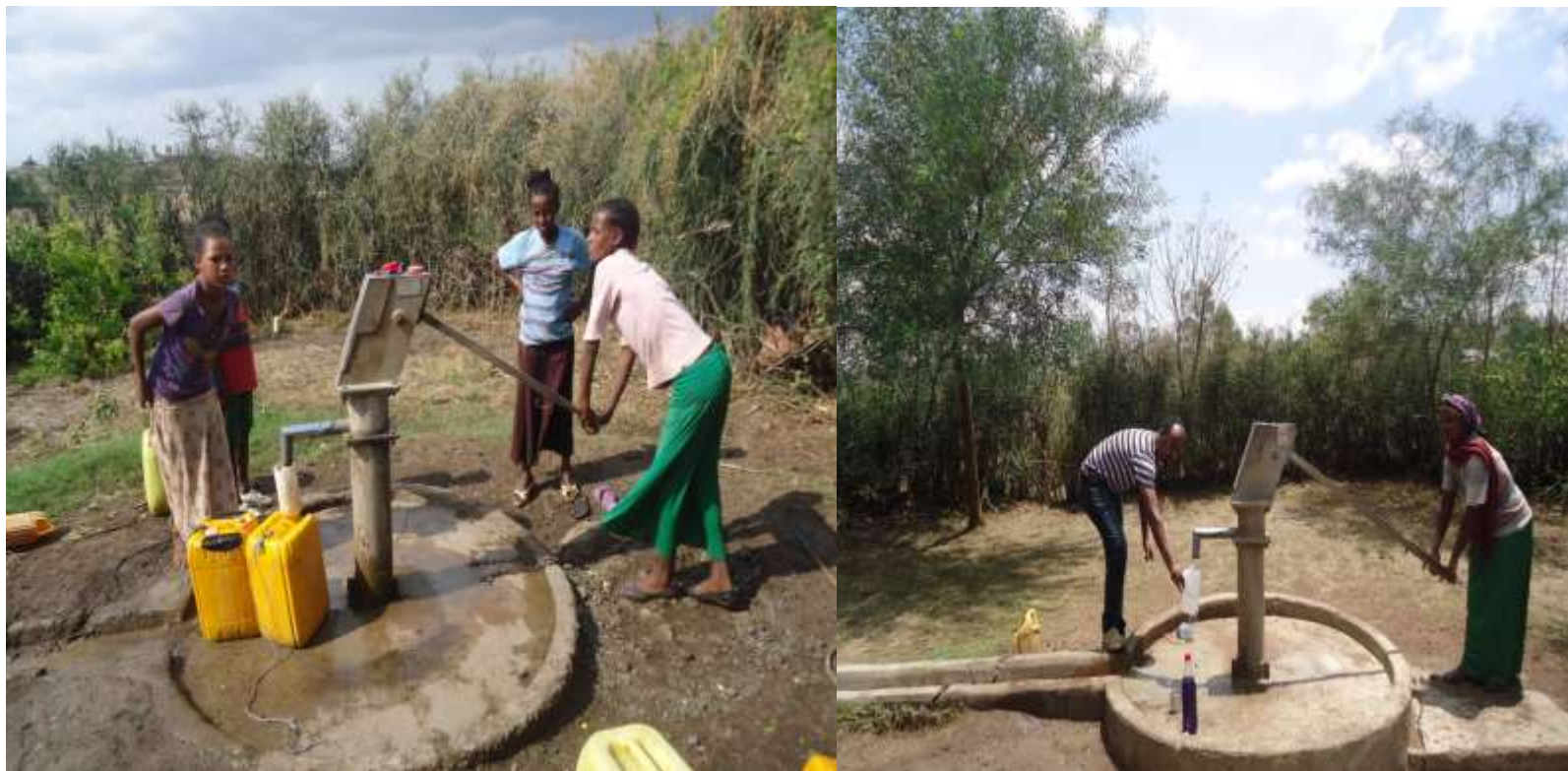
Figure 4-6:- A Poorly Constructed Shallow Well with a Cracked Apron versus Well Constructed Shallow Well
