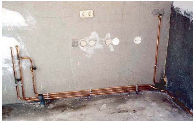
Figure 4.38. Indoor installations made of copper.
