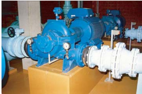
Figure 4.77. Horizontal pumps with rubber rings to dampen vibrations.
