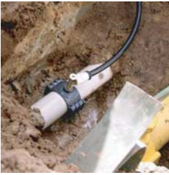
Figure 4.70. Service connection made with PE on a PVC pipe under pressure.
