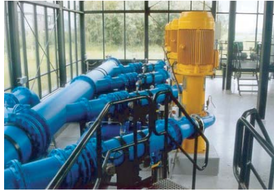
Figure 4.78. Unmanned booster pumping station.
