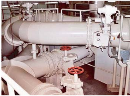
Figure 4.76. Piping in pumping station.
