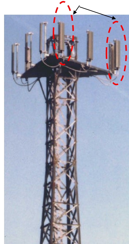
Diversity antennas for one sector (cell)
