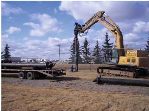
Fig. 12.9 One of a number of small wind turbine pile foundations being driven into the ground. The bevel on top of the foundation seen in the foreground is cut off before attaching the turbine baseplate. Photograph by Rob Falconer, Enmax Corporation
