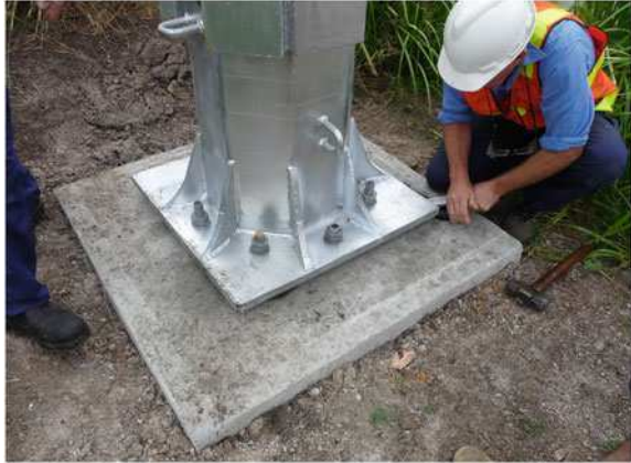
Fig. 12.8 Leveling a 5 kW wind turbine tower. This tower is hinged near its mid-height and can be easily swung up and down because the weights visible at the top of the photograph counter the weight of the turbine. Photograph by Paul Peterson
