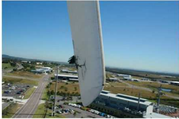
Fig. 11.14 Lightning damage at the trailing edge near the tip of a Westwind 20 kW wind turbine blade at the CSIRO Energy Centre, Newcastle. Photo courtesy of Phil May, Solartec Renewables
