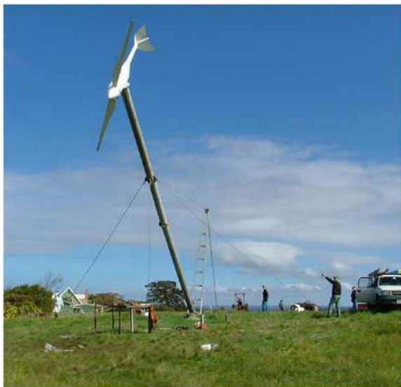
Fig. 10.10 A 5 kW turbine being raised on a guyed tower on French Island, Victoria, Australia
