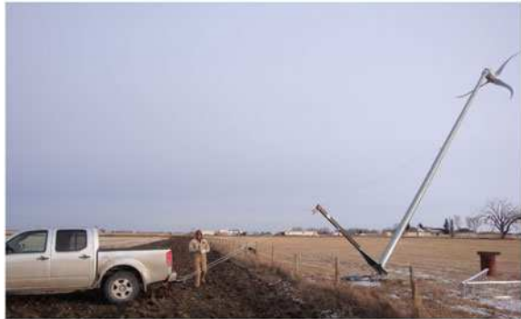
Fig. 12.7 A Skystream 2.4 kW wind turbine on a monopole tower being raised using a gin pole and winch attached to a four-wheel drive vehicle. Photograph by Rob Falconer, Enmax Corporation
