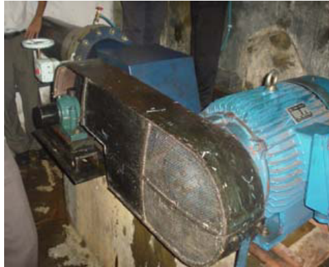
Fig. 19.2. Micro hydropower plant (25 kW).
