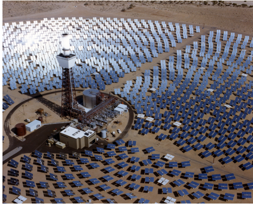
Fig. 10.15. Solar One central receiver CSP facility (courtesy of DOE/NREL).
