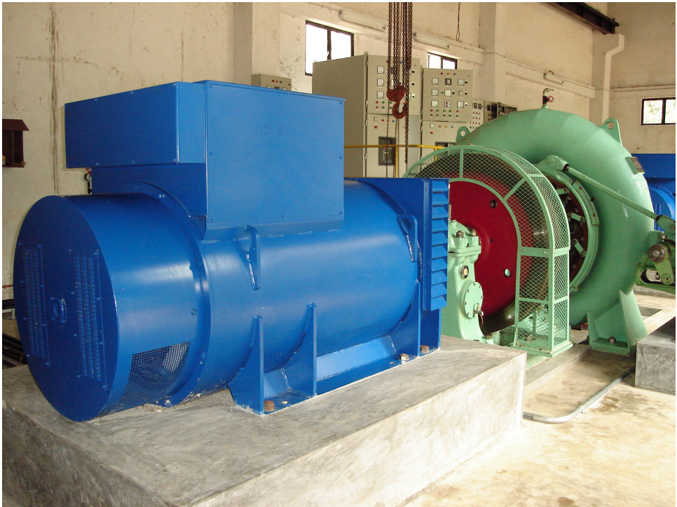
Fig. 19.1. Small hydro power plant (one unit 1250 kVA).
