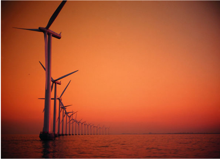
Fig. 5.30 An offshore wind farm at Middelgrunden near Copenhagen, Denmark. Each rotor blade is 36.8 m long (courtesy of LM Glasfiber, www.lmglasfiber.com )
