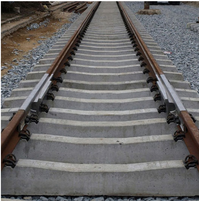
Fig. 8.5 Spring fastening of rails for the tram tracks in Prague ( http://www.prazsketramvaje.cz/view.php?cisloclanku=2010031701 )
