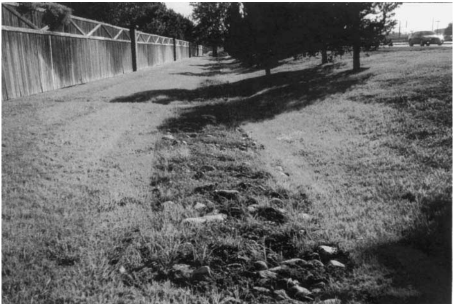
FIGURE 9.5 Infiltration trench installed along highway.
