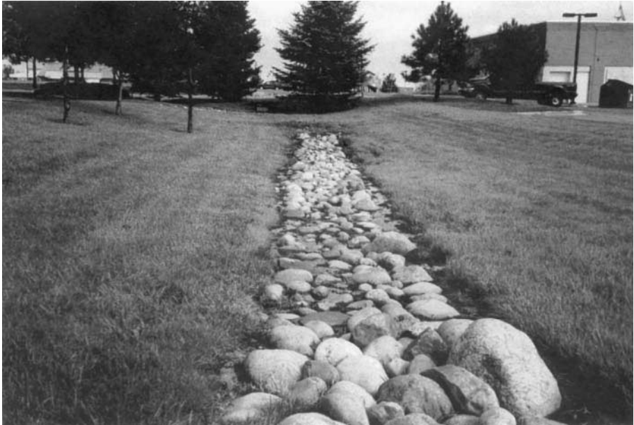
FIGURE 9.4 Infiltration trench built in business district.
