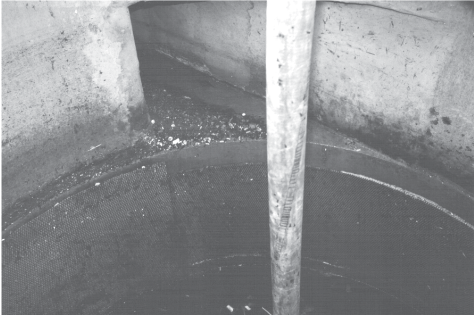
FIGURE 19.11 View of the inside of a CDS device. The unit is being drained for cleaning. The inlet culvert and the screen are clearly visible.
