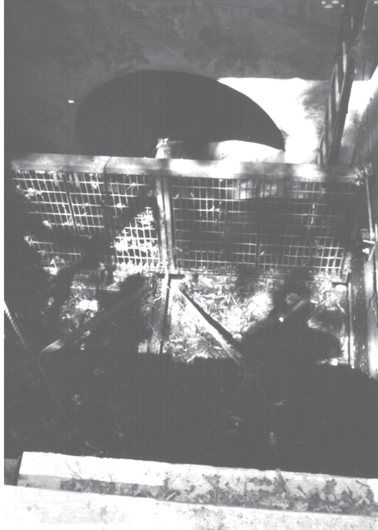
FIGURE 19.7 View inside a North Sydney Litter Control Device (LCD).
