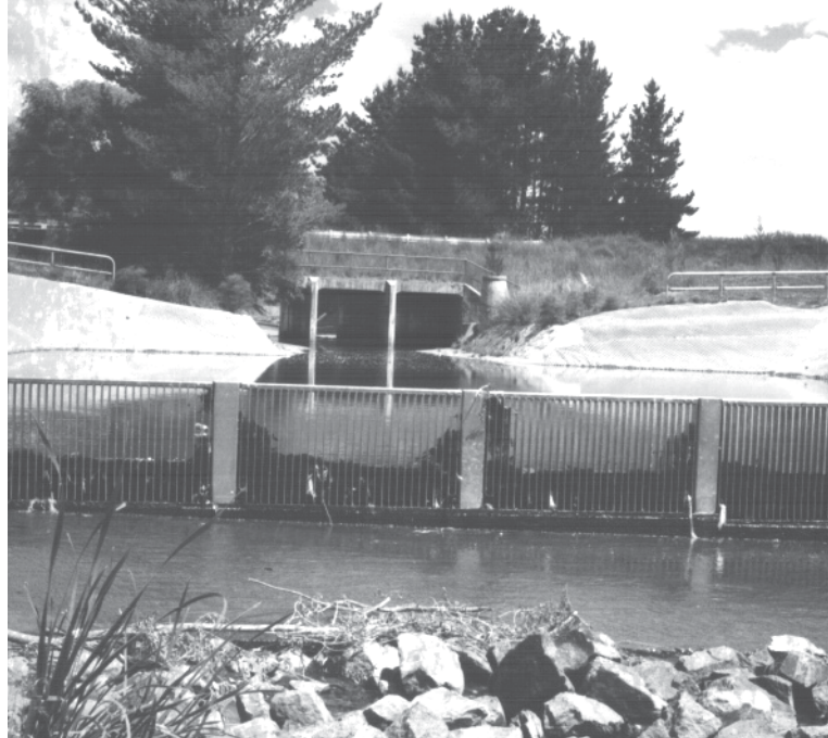
FIGURE 19.3 Typical example of blockage on a vertical screen.
