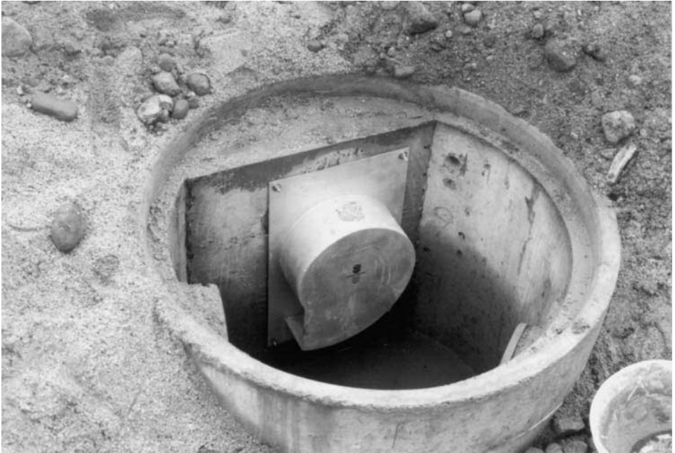
FIGURE 18.29 Plate mounted Type “SH” Vortex Valve. Design discharge of 0.42 cfs (12 l/s) under a 5-foot head, City of Portland, Maine. The “SH” unit was installed in a 4-ft. diameter manhole. Intake to the unit is on the bottom left. This unit is plate mounted as the outlet pipe is larger than the casing of the control unit. Normally, this type of unit is fixed using 3 lugs and anchor bolts or a push-fit spigot/sleeve arrangement. (From HydroInternational, PLC)
