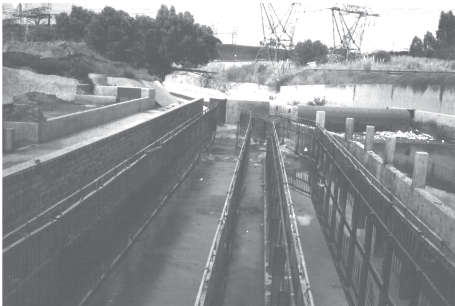
FIGURE 19.17 View of the Robinson Canal screens after cleaning. The hydraulically operated sluice gate is clearly visible on the top right-hand side of the picture.
