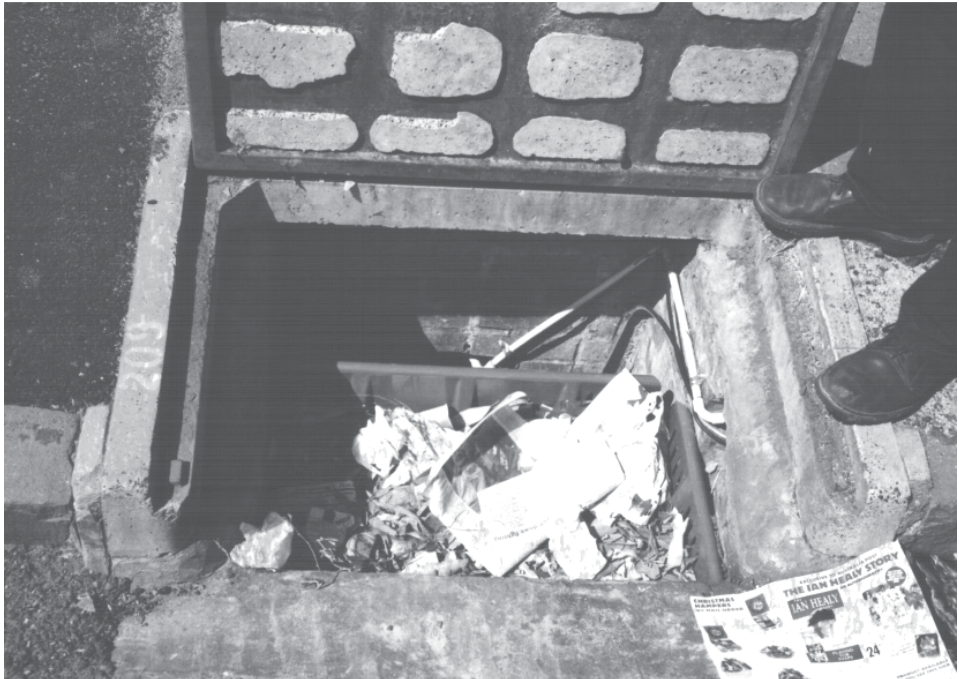
FIGURE 19.5 View of a typical side-entry catchpit trap.
