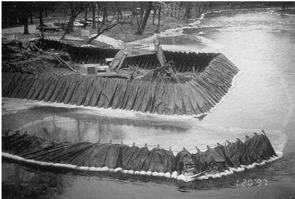
FIGURE 17.5 TRM being rolled out and installed in an urban channel. (From IECA, 1998)
