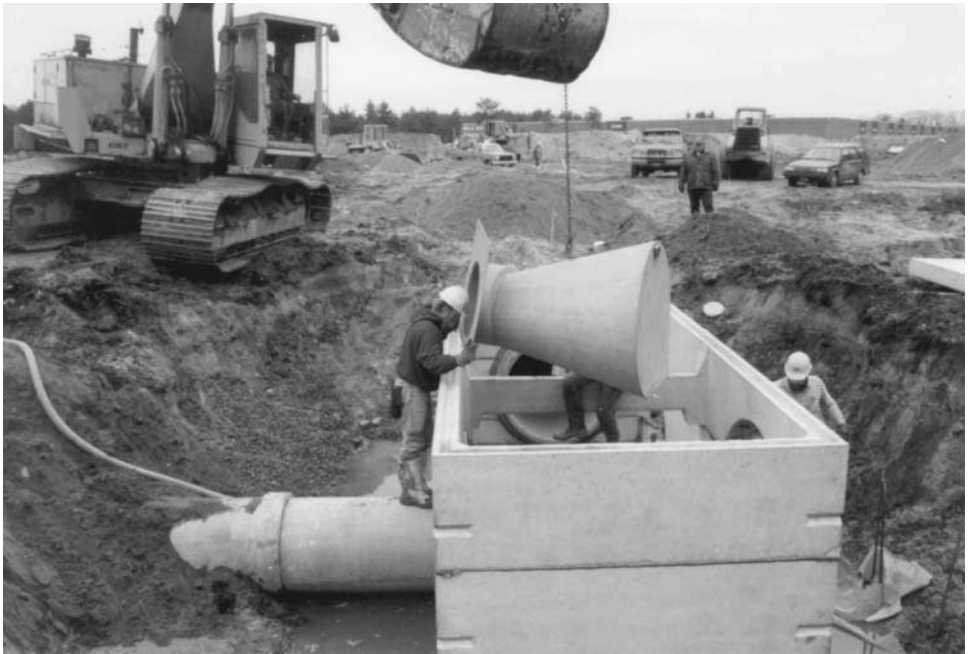
FIGURE 18.31 Type “C” Reg-U-Flo Vortex Valve. A 22-inch Type “C” Reg-U-Flo Vortex Valve discharging 15 cfs (425 l/s), installed at the Eastern Mall Office Park project in South Portland, Maine. This photograph shows the valve being lowered into place in the precast concrete control chamber. This stormwater management project was designed by H.I.L. Technology, Inc. By storing the 2-year storm within the pipes and manholes and the 25-year storm on the parking lots, the developer was able to avoid the construction of a detention pond which would have required the purchase of additional land. (From HydroInternational, PLC)
