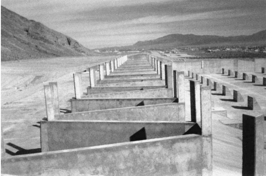
FIGURE 8.29 Emergency spillway for a regional detention basin, City of Henderson, Nevada.
