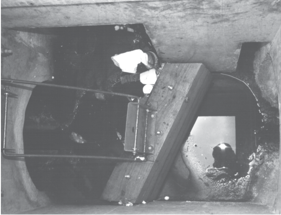
FIGURE 19.9 View of the In-line Separator (ILS). Flow from left to right.
