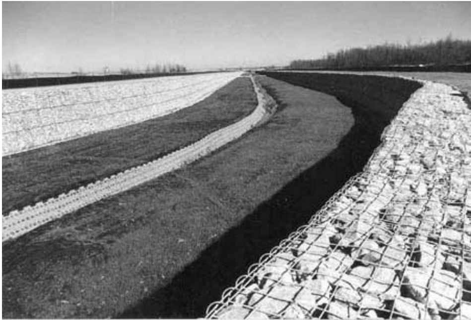
FIGURE 17.8 Grass-lined channel with gabion basket. (From IECA, 1998)
