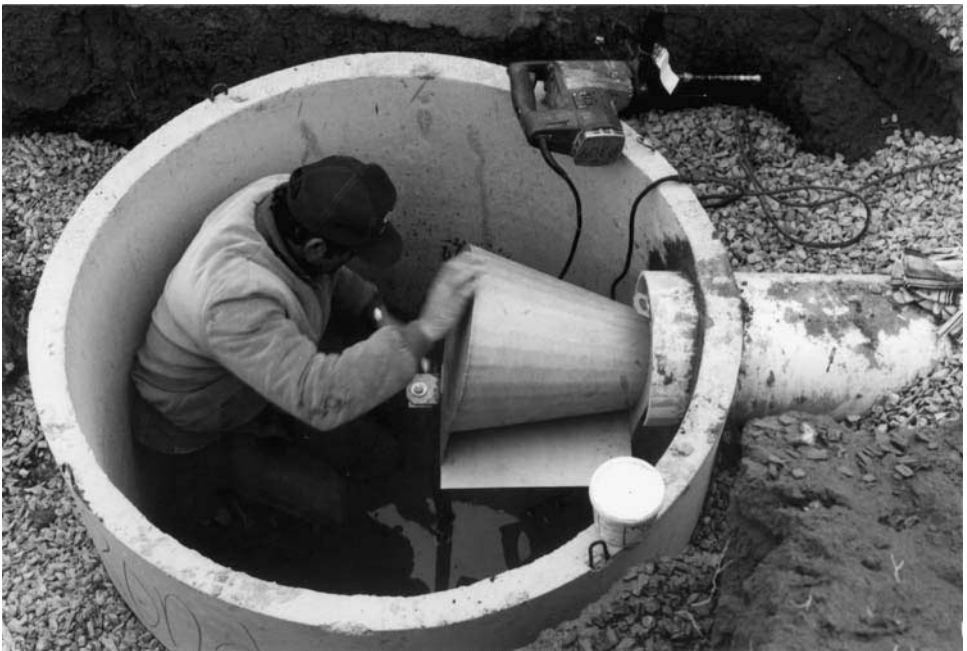
FIGURE 18.30 6-Inch Type “C” Conical Reg-U-Flow Vortex Valve. Installed in a 4-ft diameter catchbasin. This unit was supplied with a sleeve pipe which was inserted into the outlet pipe and sealed by 2 neoprene rubber “O” rings. The consultant on this project wished to maintain a silt trap so the control unit was mounted 3-feet above the base of the chamber with an additional support member to anchor the base of the cone. (From HydroInternational, PLC)
