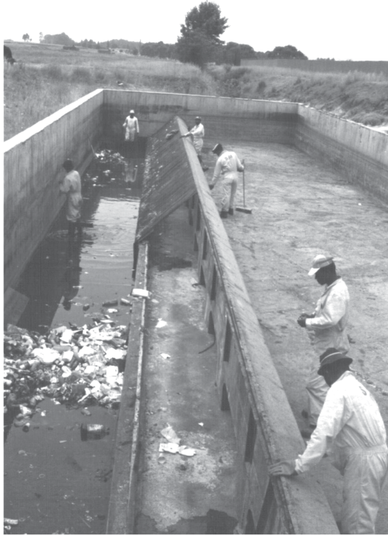
FIGURE 19.15 View of an SCS structure being cleaned and repaired. The flow would normally be from right to centre and down. The collection bin is on the left.
