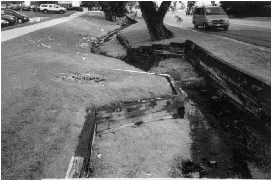
FIGURE 8.10 Parking lot detention basin using side walk as overflow diversion.
