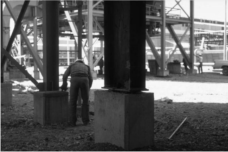
Figure 2.31 Earthquake-induced foundation settlement (Michoacán Guerrero earthquake, 1985).
