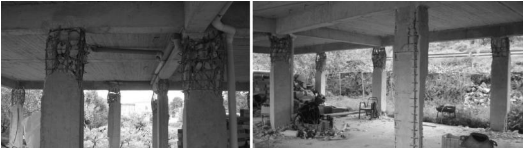
Figure 2.20 Despite complete failure of columns across the ground storey, their residual axial load capacity still supports gravity loads.
