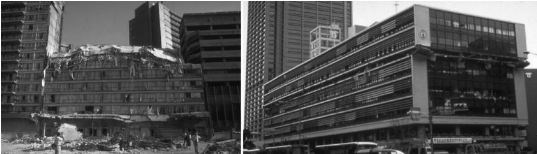
Figure 2.15 Collapse of top floors in Mexico City (1985) or of an intermediate one in Kobe (1995).
