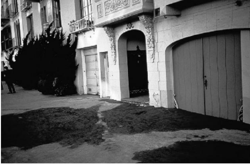
Figure 2.27 Liquefaction-induced settlement in Marina district (Loma Prieta earthquake, 1989).
