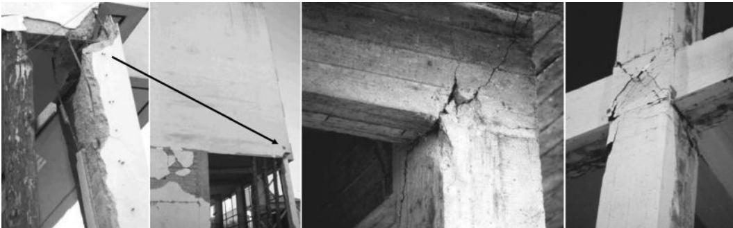
Figure 2.21 Shear failure of beam–column joints.
