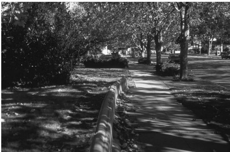
Figure 2.4 Fence offset in Hollister, California.
