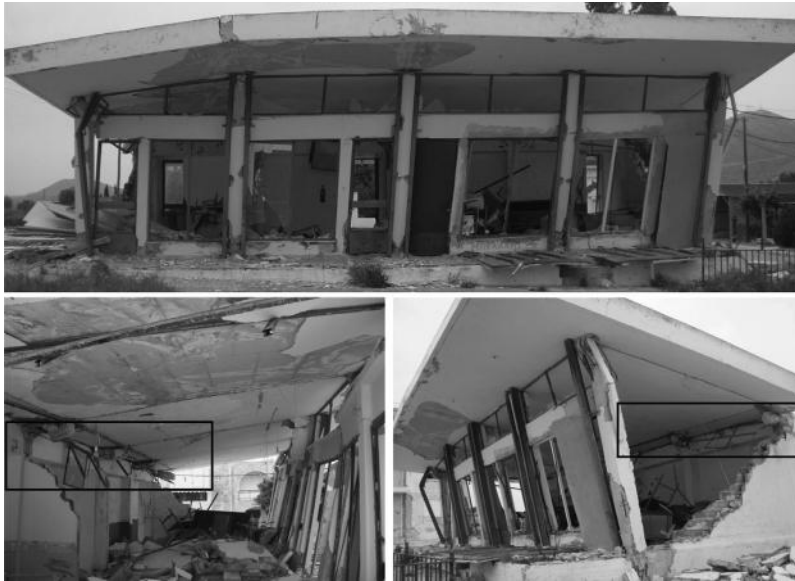
Figure 2.17 Shear failure of short columns on stiff side (inside rectangle) causes collapse of flexible side as well.
