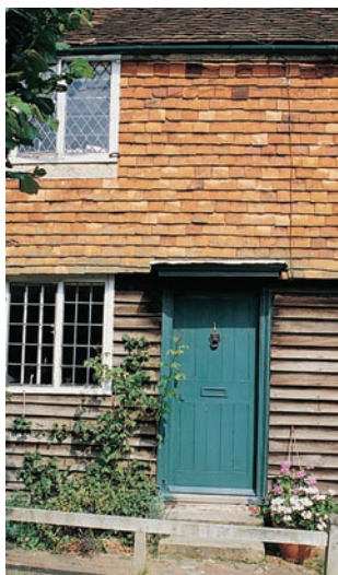
145 Black mathematical tiles applied onto brick terrace; Brighton, Sussex; terrace 1798–1807, tiles applied later.
