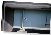
The large shear force that occurs at the support of this steel beam causes localized buckling of the beam's flange or web. To avoid this, a "stiffener" is placed along the web to maintain shape.
