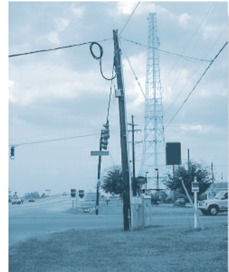
The long-term application of the cable loading on this pole has caused the pole to deform due to creep.
