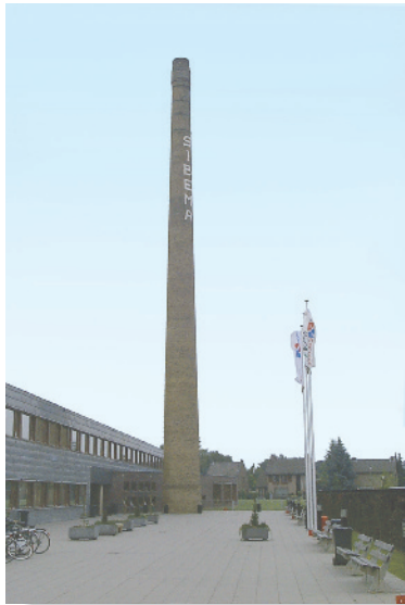
This chimney is subjected to the combined internal loading caused by the wind and the chimney's weight.
