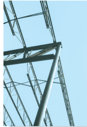
Typical example of a column used to support an eccentric roof loading.
