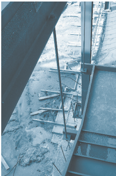
This steel tie rod is used as a hanger to suspend a portion of a staircase. As a result it is subjected to tensile stress.
