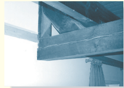
Typical shear failure of this wooden beam occurred at the support and through the approximate center of its cross section.
