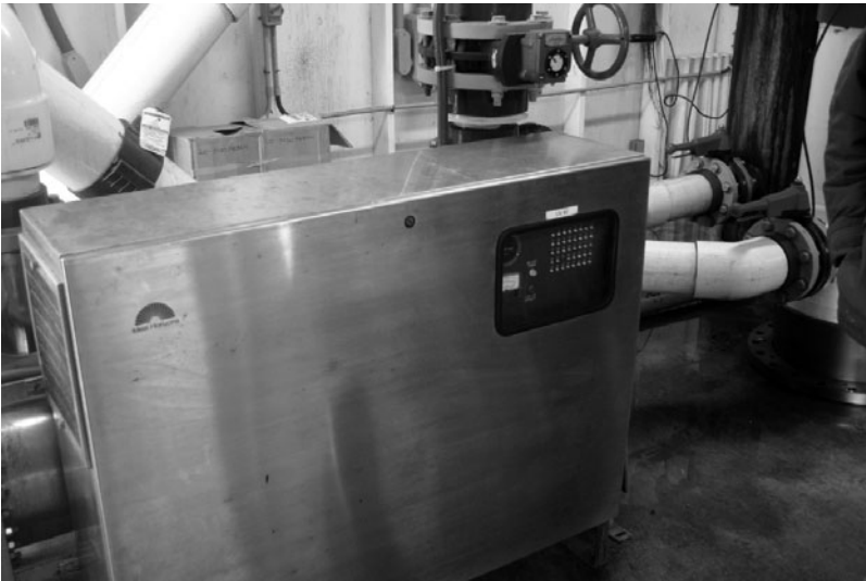
Fig. 2.26. A large ultraviolet light sterilization unit.
