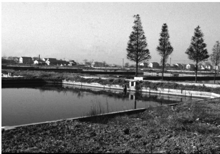
Fig. 2.2. A pond with vertical walls of brick covered with mortar in China.
