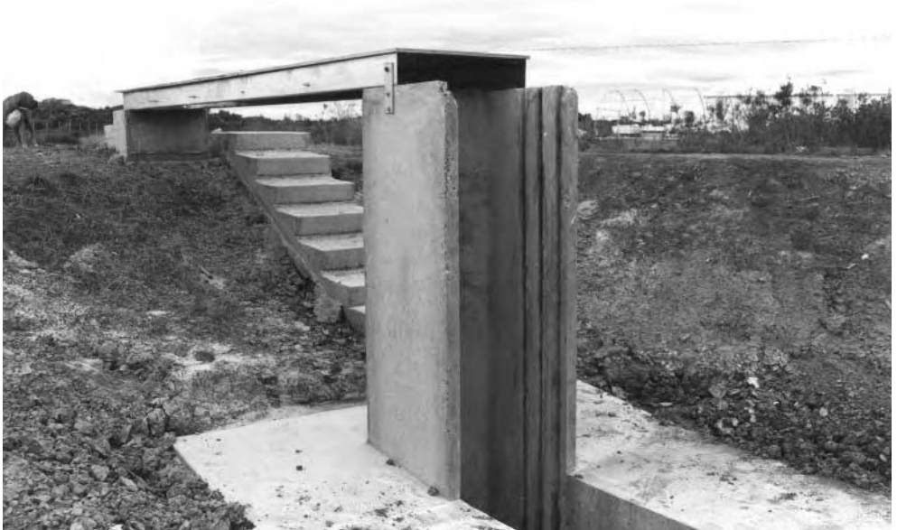
Figure 11.3. Innovation is the name of the game. Here is a monk made from the mould of a road culvert supplied after negotiation with the local concrete company. The boards weren't installed at the time of the photograph. Note also the concrete steps coming down into the pond and the concrete apron around the internal sump. This particular pond was a fry pond at a marine hatchery.
