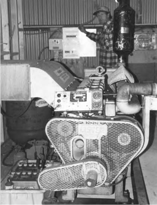
Figure 11.9. With a life span of 20 to 30 minutes for your fish, should the power go down, emergency generation capacity is essential in re-circulation systems, or any aspect of aquaculture that is reliant on power for its aeration.
