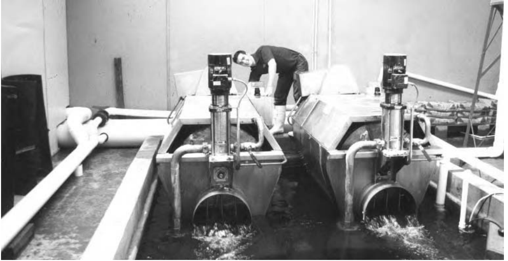
Figure 11.8. A pair of drum filters in a re-circulation system. The organic solids in suspension are removed and the water is returned to the system.
