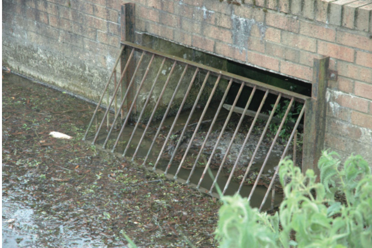
Figure 10.8 Simple weir with wooden boards.
