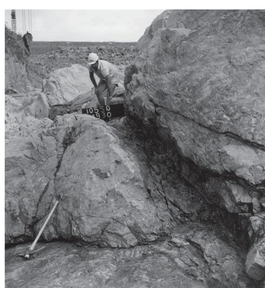
Excavation of sheared zones prior to filling with dental concrete in the cutoff foundation
