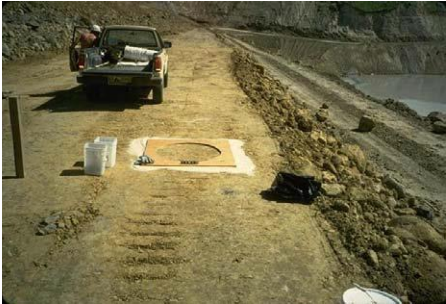
Compacted rockfill placement in relatively thin controlled lifts for heavy roller compaction
