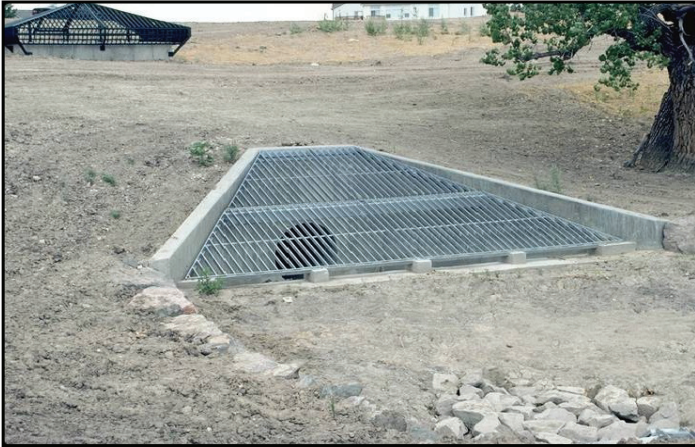
Photograph 7. Detention pond outlet pipes often require debris/safety racks, which should be sloped and have large surface areas to reduce the risk of a person being pinned against the rack and to enable debris to rise up on the rack as the water level in the pond rises.
