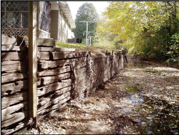
Photograph 5. The hazards in this situation are striking—unstable, high vertical wall, little separation distance from house to channel, undersized channel with high-velocity flows, and home in floodplain.
