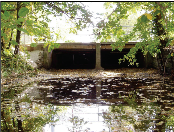
Photograph 44. Transitions from open channels into long underground culverts and pipes must be carefully evaluated and will often require a rack at the inlet.
