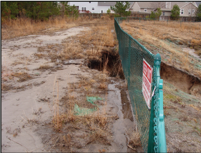
Photograph 16. Banks of wet pond that were not stabilized with groundcover have eroded, resulting in a gully through which children could gain access to the pond.
