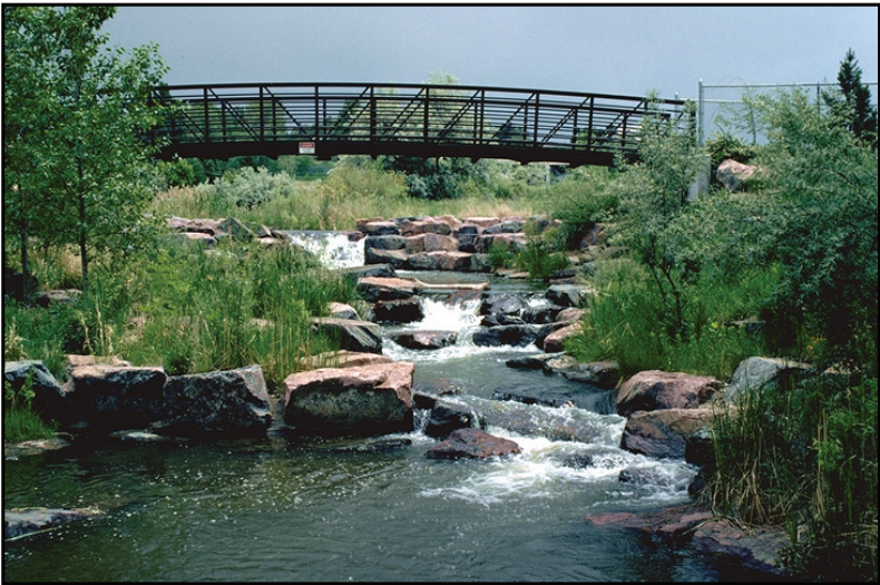
Photograph 40. Pedestrian bridge across engineered urban channel. Note fencing and railings to protect trail users.
