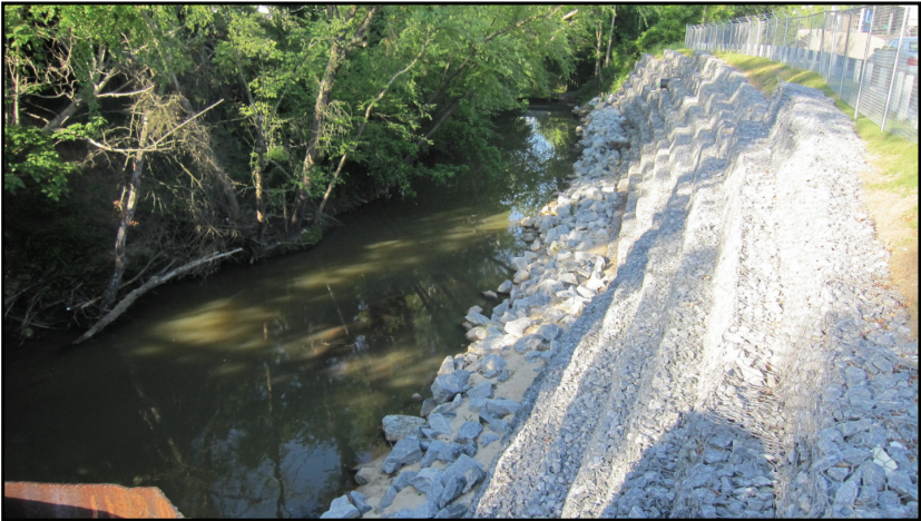
Photograph 48. At this steep gabion wall with rock toe protection, separation from the parking lot is essential and is provided by both guardrail and fence.
