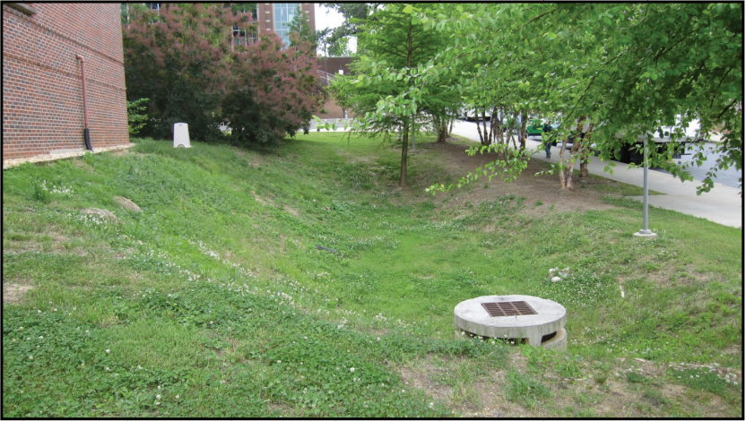
Photograph 11. Traditional dry pond with an outlet structure that has small orifices and a grate on overflow.
