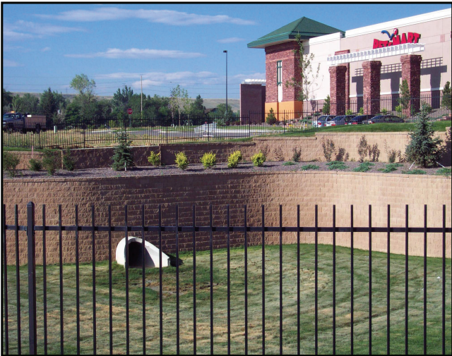
Photograph 20. Storage facilities with vertical retaining walls or steep slopes absolutely require a safety fence or other means to keep the public away from the walls, and terraced walls are encouraged, especially near the top.
