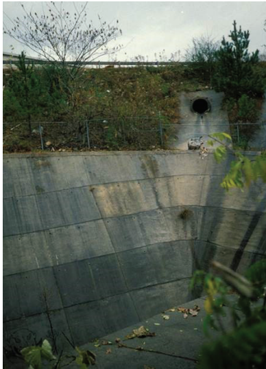
Figure 2. Dry Detention Basin, Culvert and Rundown with Safety Concerns Due to Steep Side Slopes and No Egress or Escape Route
