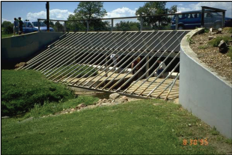
Photograph 8. Large sloping rack discourages entrance into long multibox culvert. (Note: People behind the rack are inspectors.)
