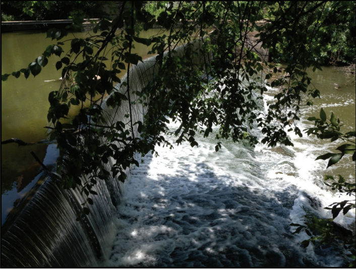
Photograph 45. Low-head dams in urban settings can be very dangerous, but various techniques can be used to eliminate the “keepers” (reverse rollers) often found on the downstream side of the dam.
