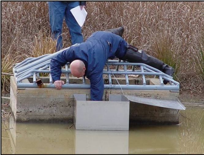
Photograph 12. An outlet structure that was not designed to facilitate maintenance, creating a risk of injury to maintenance workers. Maintenance is essential to promote economic, environmental and community benefits.
