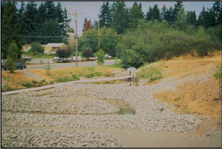
Photograph 24. Sinuous low-flow channel in created wetland (under construction) promotes water quality enhancement while also addressing public safety with good footing, shallow depths and safe outlet structure.
