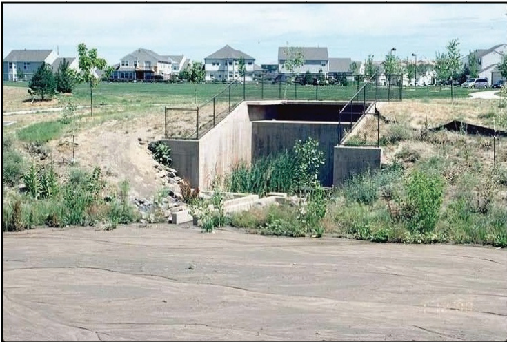
Photograph 10. Fencing is necessary (and required by local building code) at this outlet structure headwall. Fencing and railings should be visually appealing.
