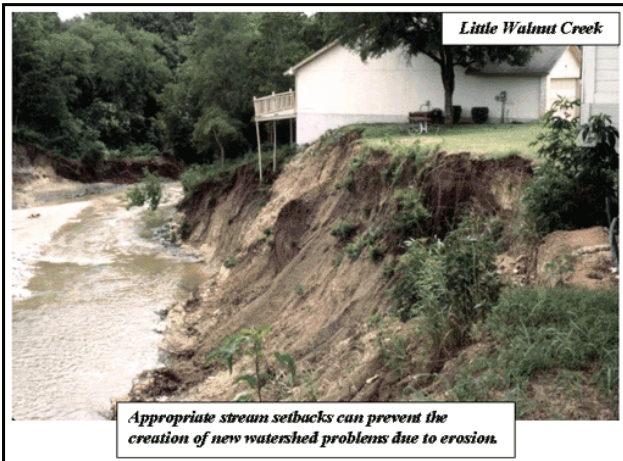
Photograph 4. Sometimes urban stormwater improvements—such as bank stabilization in this case—are urgently needed to protect the public. Attractive, environmentally sensitive stabilization consistent with local conditions can enhance public safety by promoting more public interaction with the channel.
