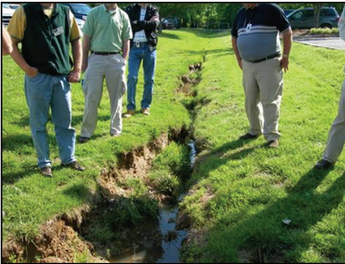
Photograph 29. Erosion caused by improper velocity check for liner has created a tripping hazard.
