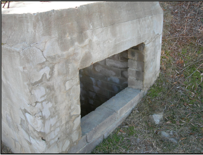
Photograph 9. Unprotected opening in outlet structure, which allows children access to the interior, where they could be trapped or injured.
