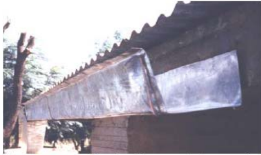
Square gutter fixed without splash-guard.
