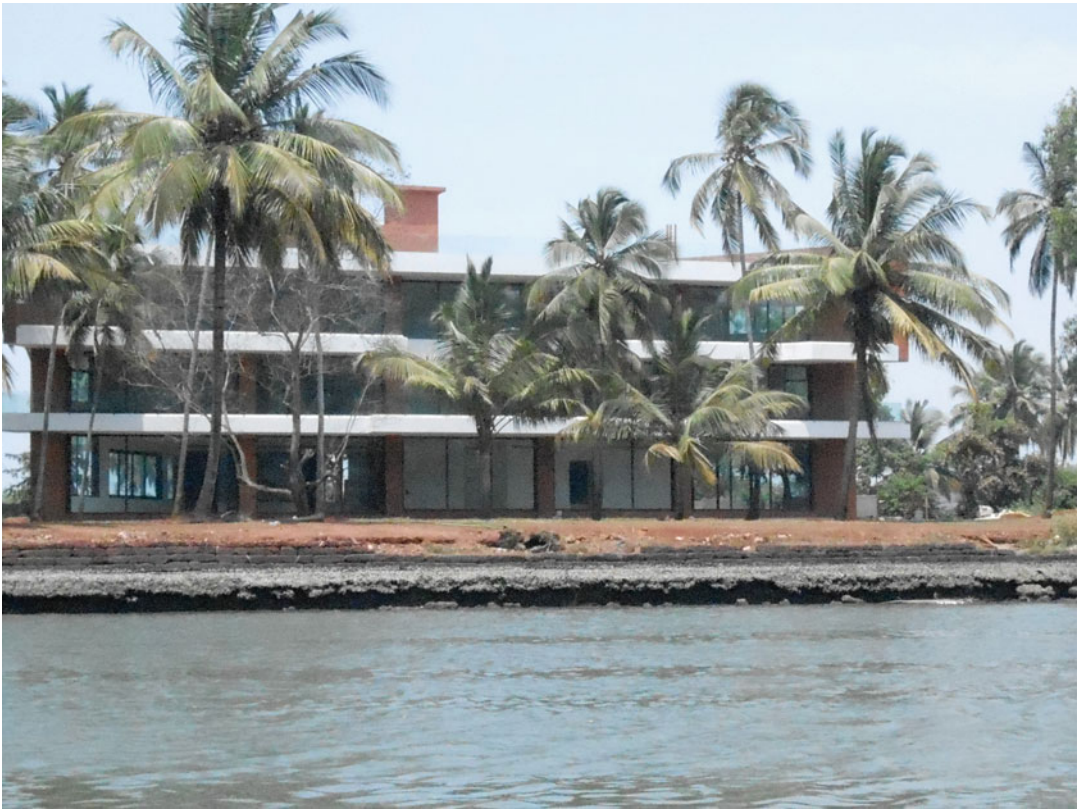
Fig. 10.14 A hotel under construction on the Goa coast ( 15^{\circ}29'5.1''\text{N} and 73^{\circ}47'40.9''\text{E} ) [Photograph taken on 04.04.2013 by Ms. Ankita Mitra (environmentalist)]
