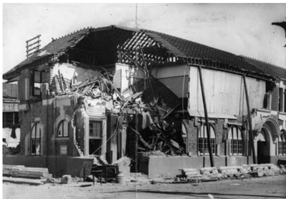
Fig. 7 Post office damaged by the 1931 earthquake in Hastings, New Zealand Courtesy of Alexander Turnbull Library
