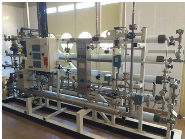
Fig. 3 View of the reverse osmosis device to treat deionized water to obtain purified water
