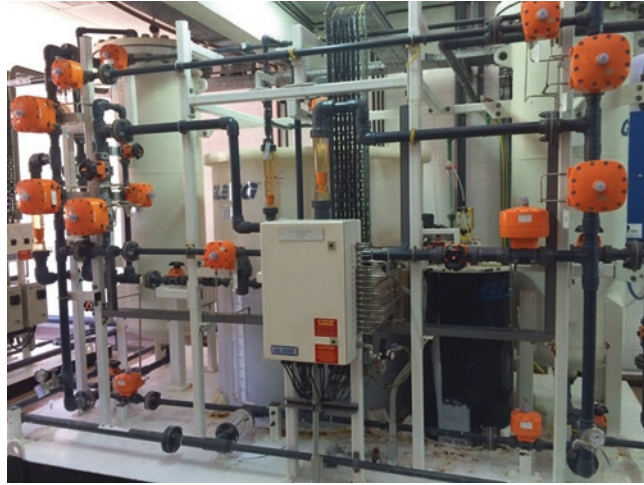
Fig. 2 Photograph of the skid holding the water deionization equipment
