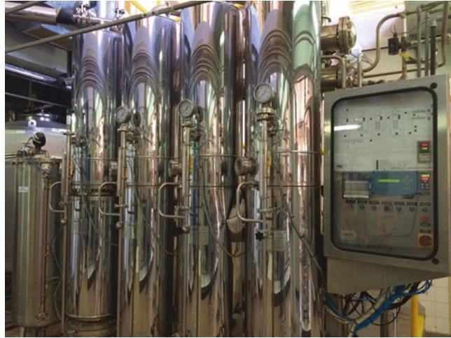
Fig. 4 Multiple effect distillation equipment to process pure water to collect water “for injection” quality
