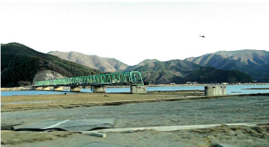
Fig. 1.13 Shin-Kitakami Ohashi Bridge across the Kitakami River at 4 km from the mouth. Its northern sections are washed out by the 2011 Tohoku tsunami. Photo by H. Tanaka
