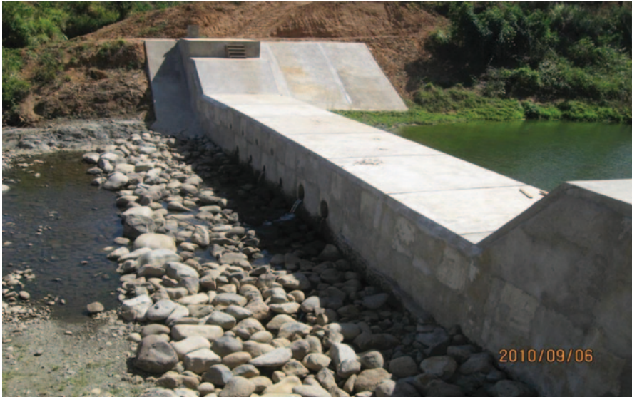
Fig. 4 A dam constructed to minimize flooding in the upper Nadi Basin in Fiji. Note low water levels and impassability to freshwater fauna. Photo credit: Vinesh Kumar
