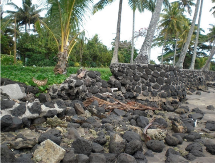
Fig. 5.6 Damage coastal defences in Independent Samoa
