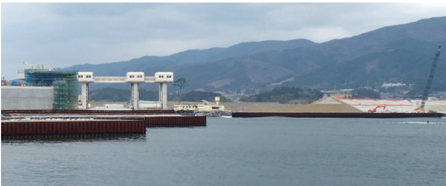
Fig. 18.5 Seawall and coastal dike construction by the Kesen river estuary in Rikuzentakata City (Iwate prefecture) (Photo taken in March 2016 by V. Santiago-Fandino)
