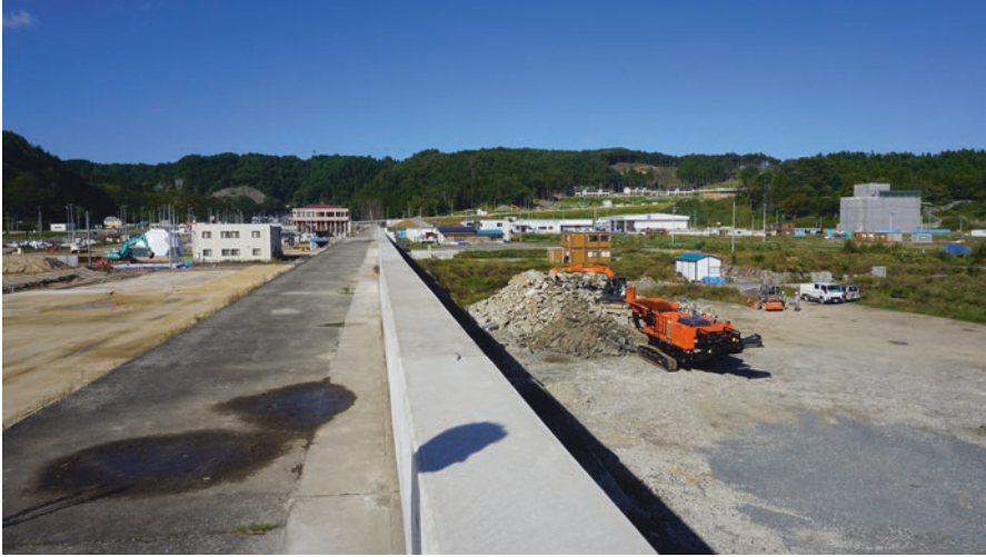
Fig. 4.2 Elevation of the remaining seawall in Taro District (Miyako City) (Photo by the author, October 2015)
