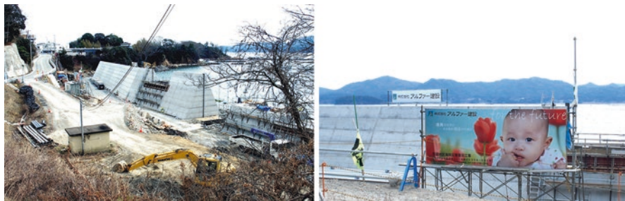
Fig. 18.7 Seawall construction and billboard at Shimizuhamama town (Miyagi prefecture) with the English message “for the future” (Photos taken in March 2016 by V. Santiago-Fandino)
