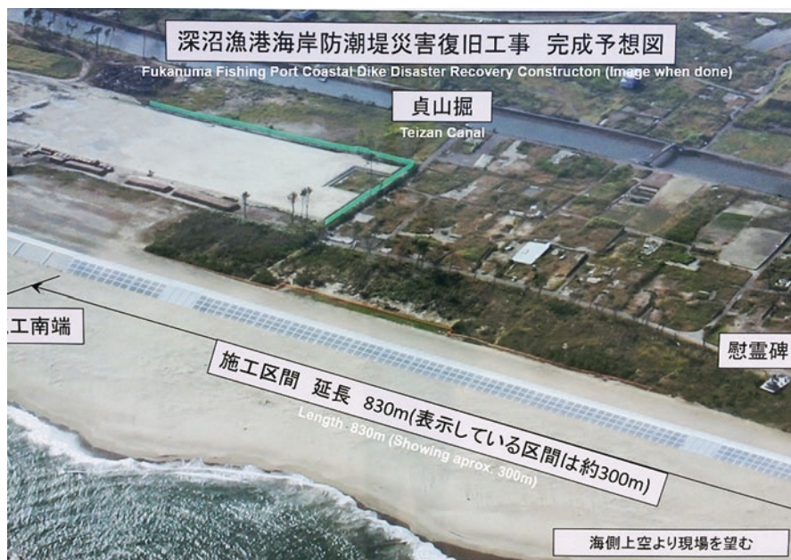
Fig. 18.10 Panel of an aerial view of the recently built 830 m long sea dike at Sendai (Miyagi Prefecture) (Photo taken in July 2015 by E. Mas)
