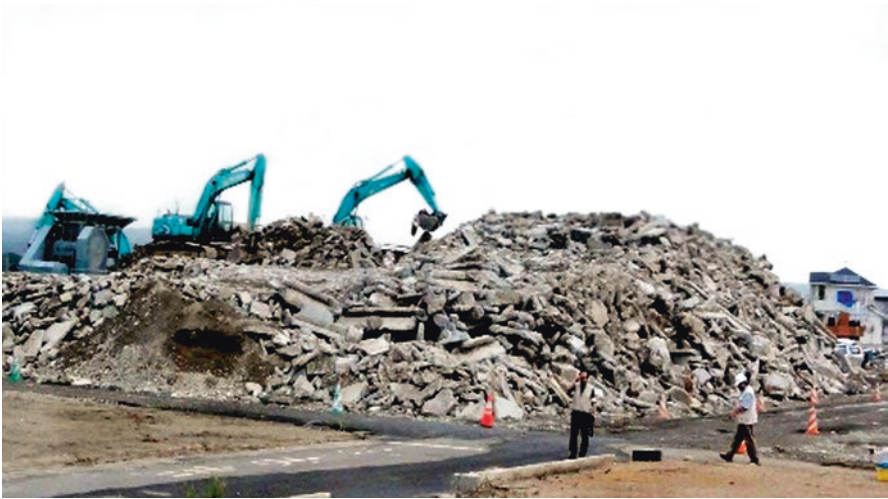
Fig. 5.9 Temporary storage of concrete rubble in Natori, Miyagi Prefecture (Photo by T. Norton June 2011)
