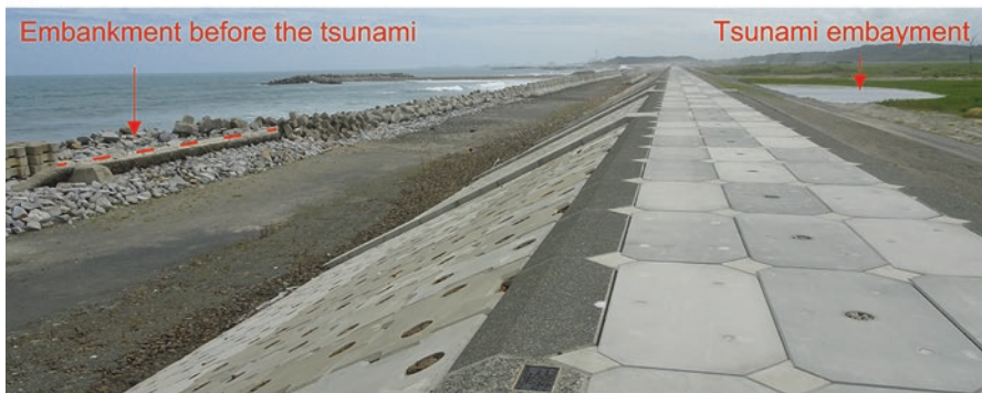
Fig. 22.10 Oblique photographs of the reconstructed embankment in cases without and with setback. (a) Without setback (taken at the location between HL No. 11 and HL No. 9, looking southward). (b) With setback (taken at the location between HL S5 and HL S4, looking southward)
