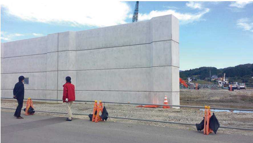
Fig. 5.22 Seawall being constructed in Kesenuma area, height approximately 10 m (Photo by T. Norton Aug. 2015)
