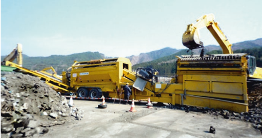
Fig. 5.12 Debris sorting processing in Otsuchi district using a rotation sorting machine, Iwate Prefecture (Iwate Pref. 2015)
