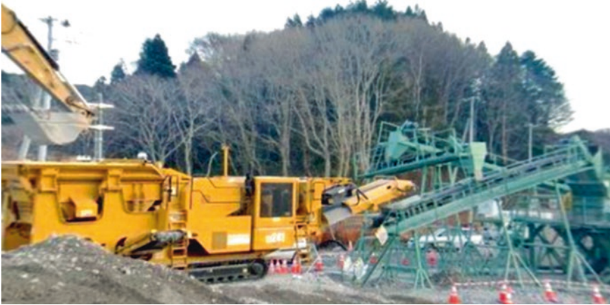
Fig. 5.11 Treatment facility for concrete debris in Yamada town, Iwate Prefecture (MOE 2012)
