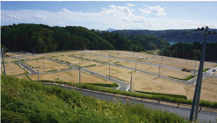
Fig. 4.3 The parcelled lots await the beginning of the construction work (Author, October 2015)
