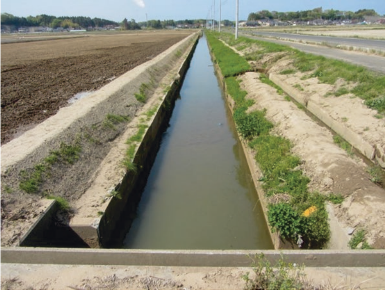
Fig. 14.13 Soma, landward of Matsukawa-ura Lagoon, Fukushima Prefecture. See Fig. 14.1a for site location. Restoration and reconstruction of drainage ditches, 2.6 km from the shoreline, as observed 10 May 2013 (Photo Yuichi Nishimura)
