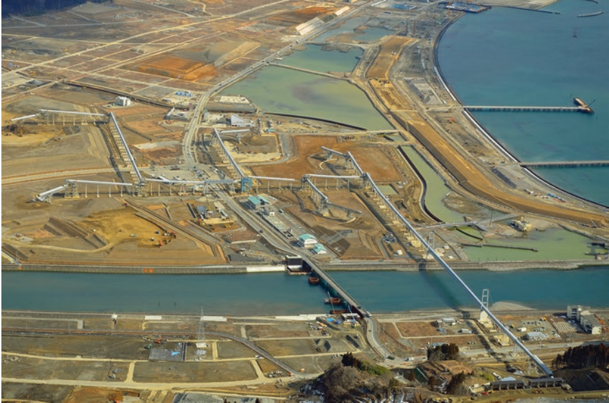
Fig. 18.4 Aerial view of Rikuzentakata's reconstruction process showing the largest conveyor belt ever constructed (tube-like structures on each side of the river banks) to deliver dug soil from the near mountain used for ground lifting and sea dike construction ( upper left and center by the shoreline). Tsunami waves destroyed the city and flooded deep inland (Photo taken in February 2015 by E. Mas during a joint reconnaissance flight with the Sendai Coastal Division of the Ministry of Land Infrastructure and Tourism (MLIT))
