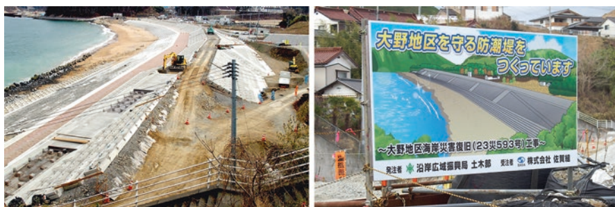
Fig. 18.8 Coastal dike construction and billboard at Ohnohama beach (Miyagi Prefecture) with the message “we are now building the seawall to protect Ohno District” (in Japanese) (Photos taken in March 2016 by V. Santiago-Fandino)
