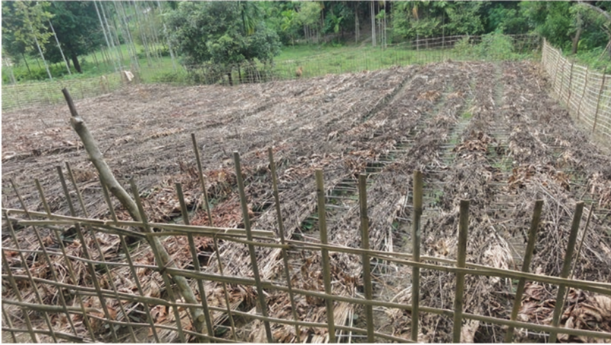
Fig. 3.4 Pan boroj immediately after planting. The roof and walls are yet to be constructed
