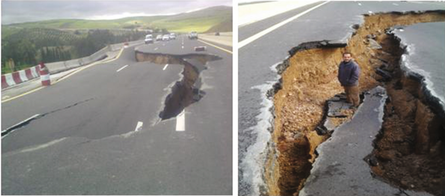
Photo 1. Deformation of the pavement body
