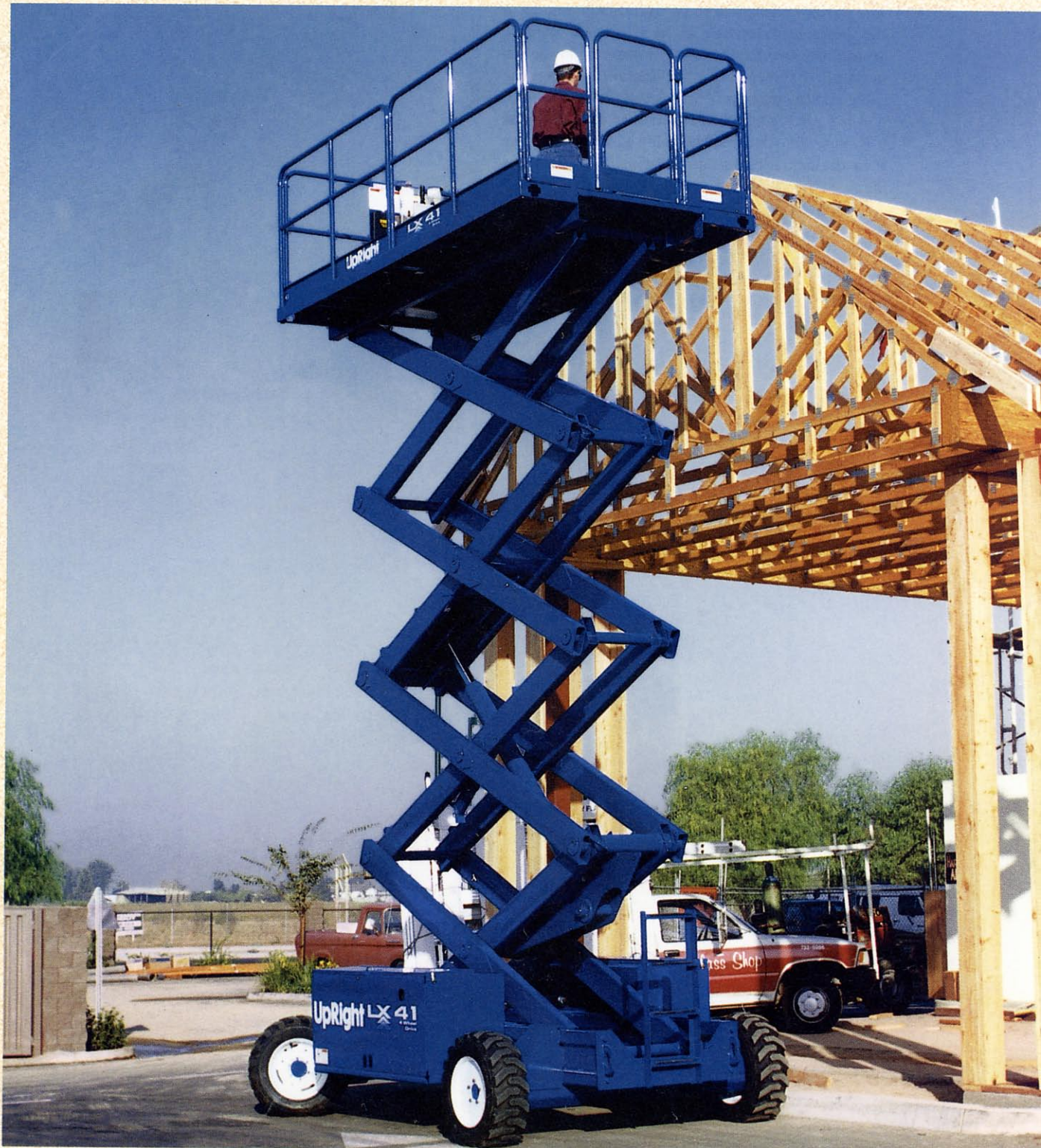
The analysis of multi-link structures which change configuration is generally best handled by a virtual-work approach. This construction platform is a typical example.
